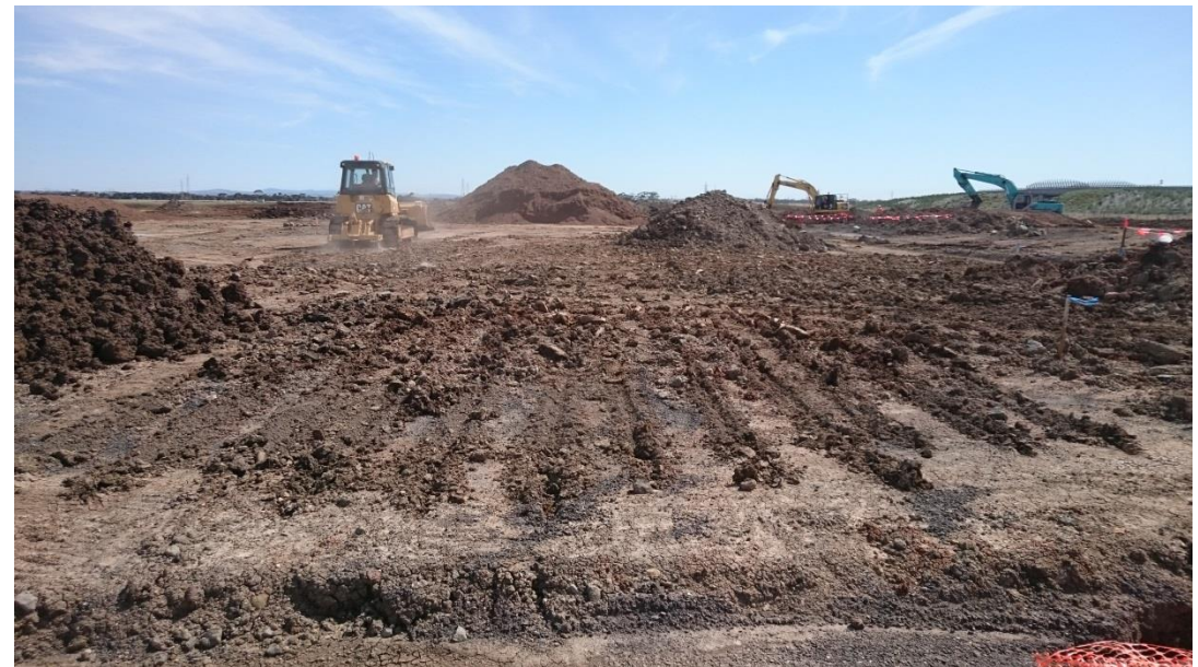
Stage 1: dozer ripping layer 6 prior to placing layer 7 in grid M1 and M2
