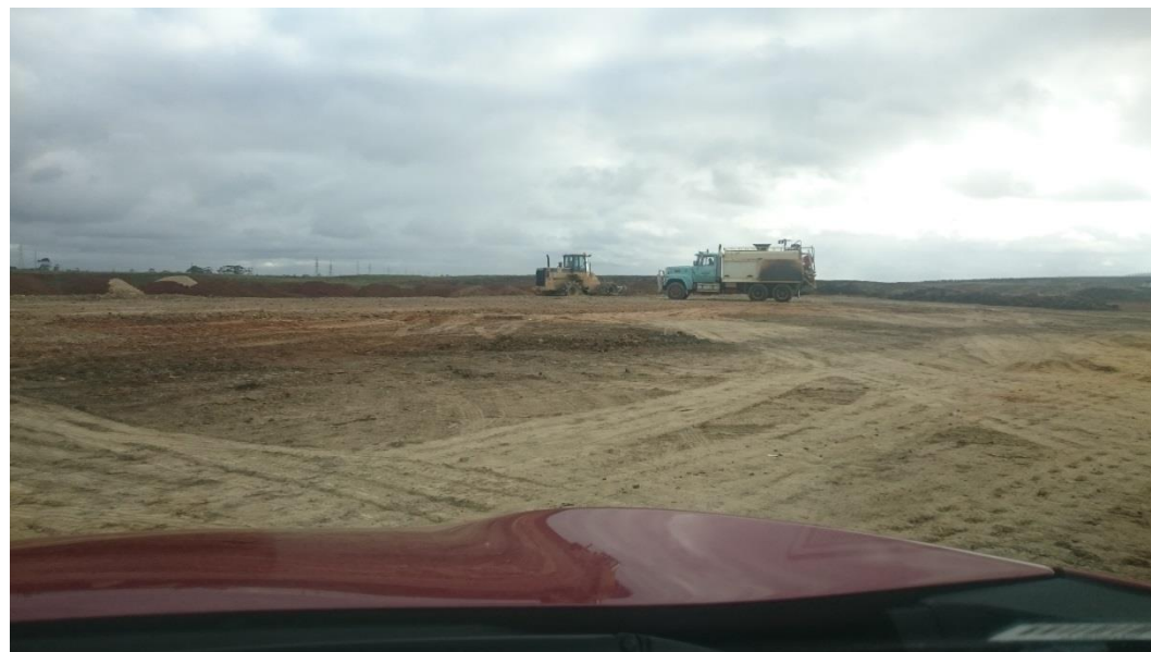
Stage 3: compactor placing layer 3 whilst being moisture conditioned in grid E5, E6, F5, F6, G5 and G6
