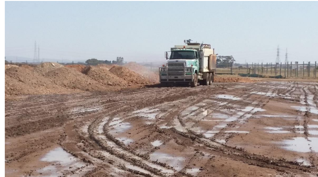
Stage 4: Moisture conditioning of subgrade and stockpiled material in grid O3, O4 and O5
