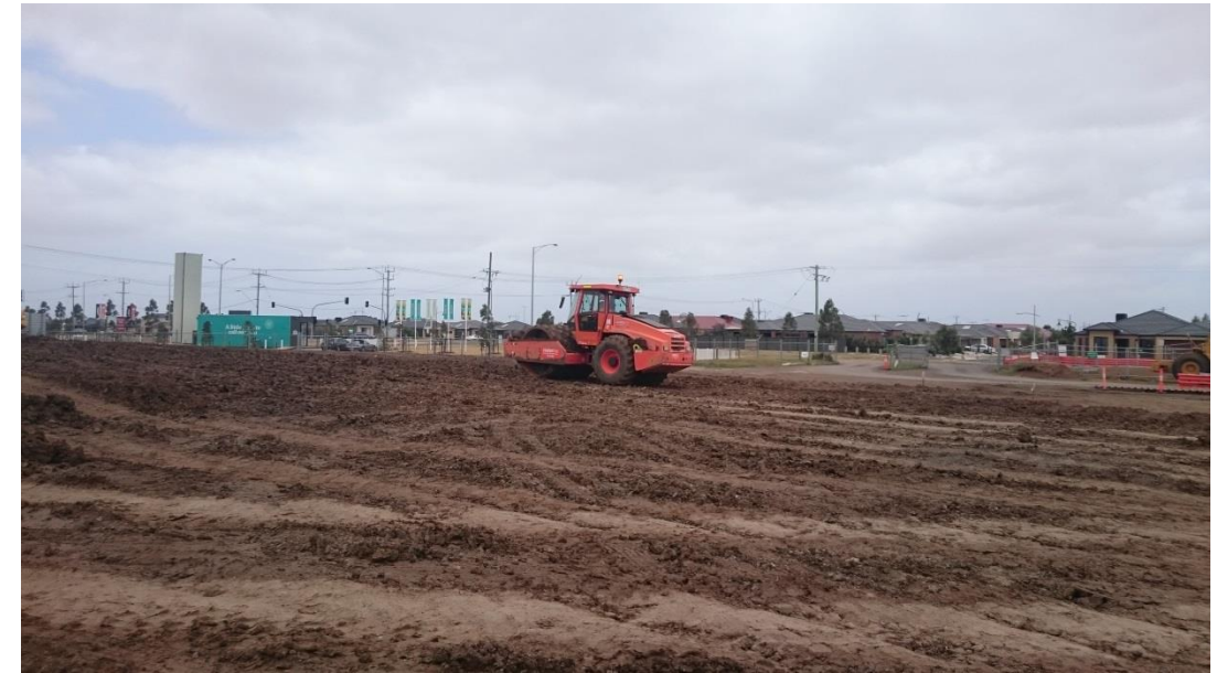
Stage 1: pad foot roller used on layer 7 in grid O1 (North) and O2 (South)
