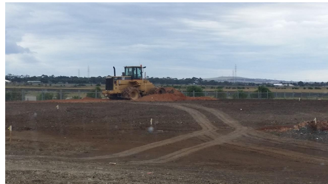
Stage 3: placement and compaction of layer 3 material in grid A5 (N) and A6 (S)
