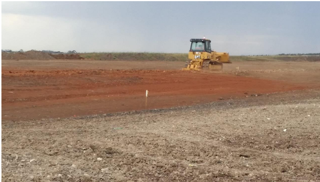
Stage 3: scarifying of layer 3 material in grid B5 (NE), B6 (SE), C5 (N), C6 (S), D5 and D6 (S)
