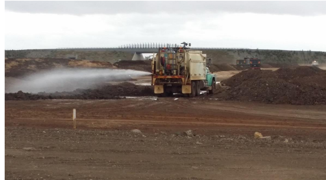
Stage 4: Moisture conditioning of layer 1 and stockpiled material prior to placement of layer 2 in grid H5 (NE), H6 (SE), I5 (N) and I6 (S)
