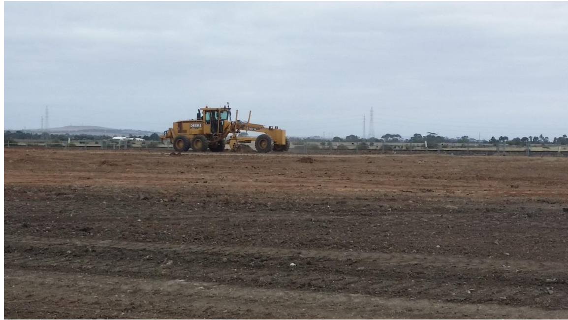
Stage 3: Grading of pad in grid B5, B6, C5, C6, D5 and D6 .
