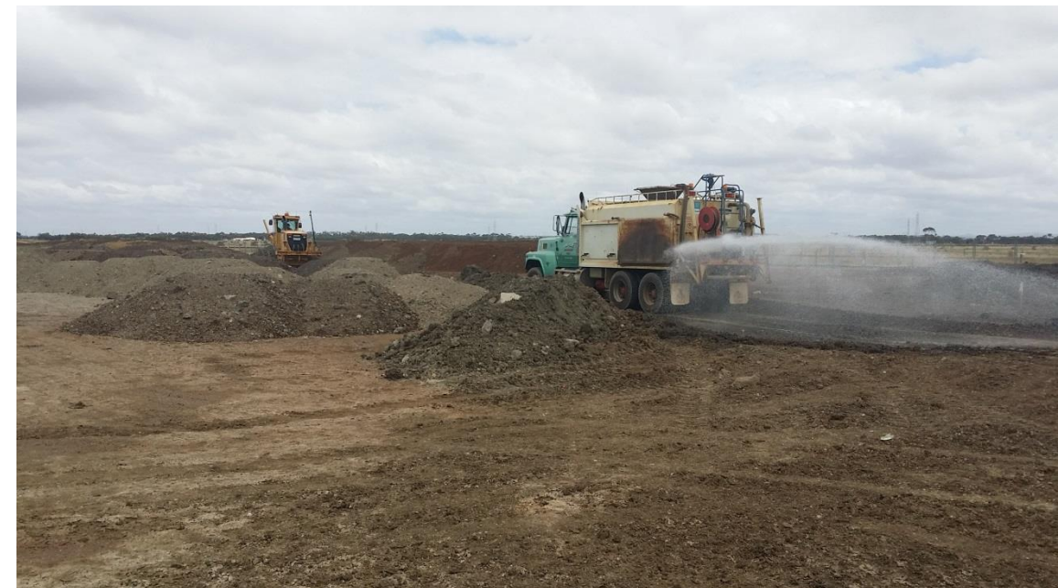
Stage 4: Placement of previously stockpiled material by grader in grid J6, K6 (S), L6 (S), M6 (S) and N6 (S).
