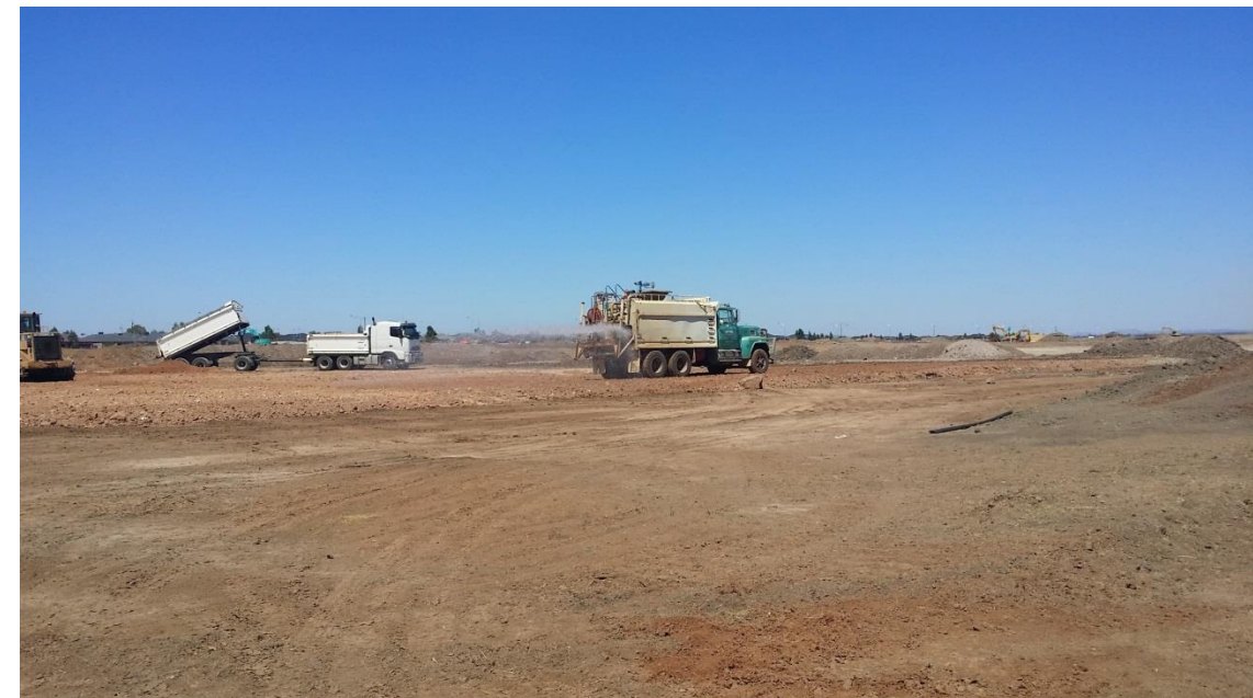
Stage 4: Moisture conditioning of placed layer 1 material in grid O4 and O5
