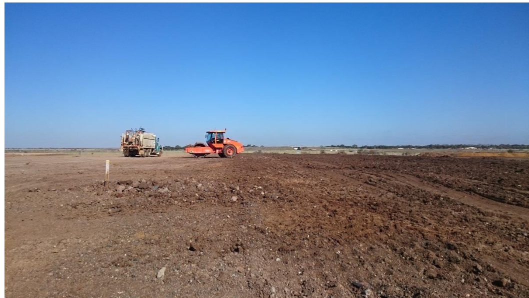
Pad foot roller and water cart on layer 4 in grid A4, B4, C4 and A5, B5 and C5
