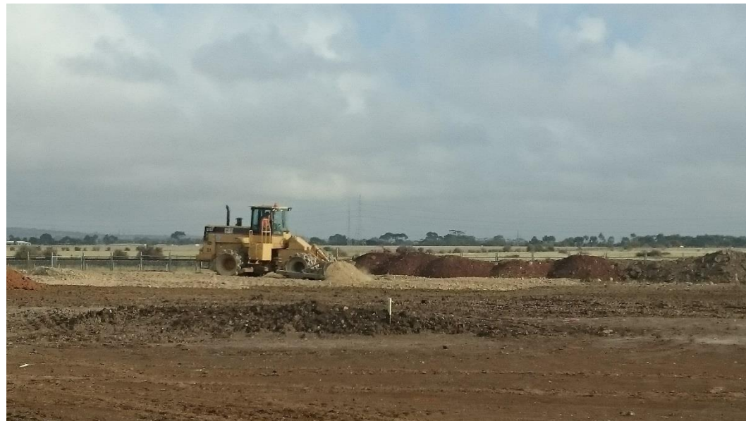
Stage 3: compactor placing layer 3 whilst being moisture conditioned in grid B5, B6, C5, C6, D5 and D6
