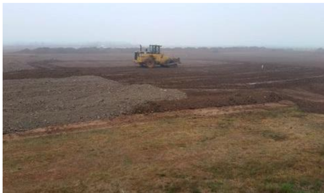
Compactor roughing up/compacting layer 2 - C5 (north), C6 (south-west), B6 (south-east), and B5 (north-east).
