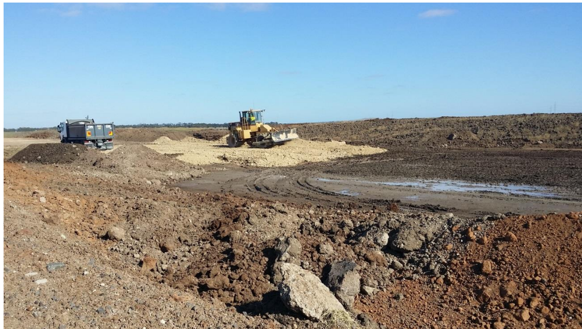
Stage 4: Placement and compaction of layer 1 material by CAT compactor in grid J5, J6 (S), K5 and K6 (S)
