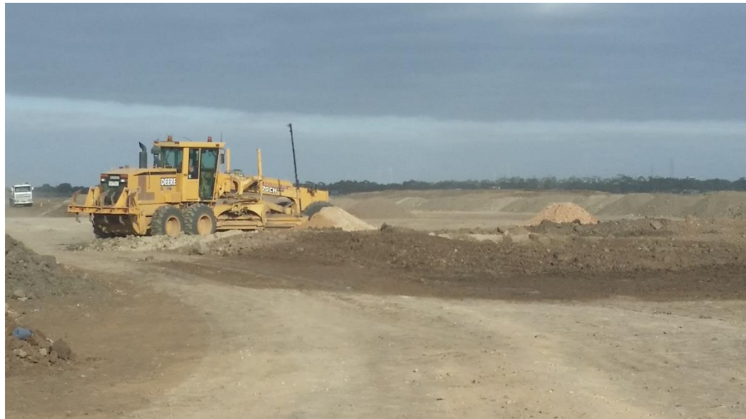
Stage 4: Filling in of uneven surfaces on layer 1 by grader in grid N4 and N5
