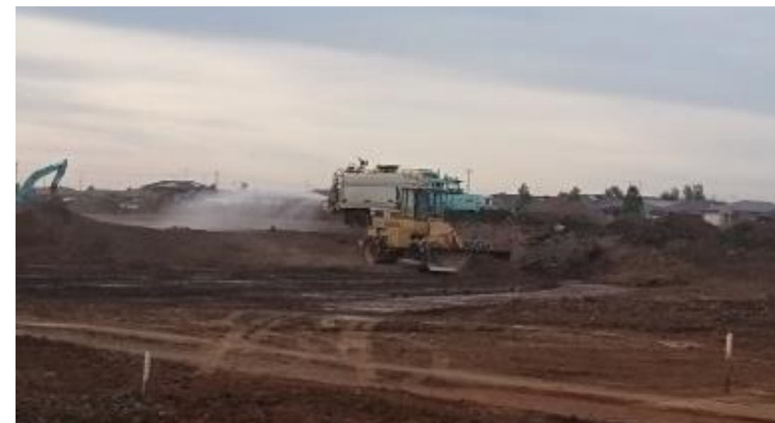
Water cart moisture conditioning the stockpile and compactor levelling layer 1 in grid G4 (Centre to East) and H4 (West, North-West and South-West)
