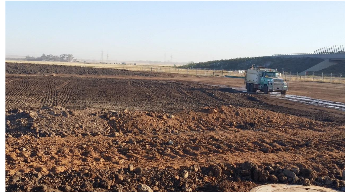
Stage 4: Moisture conditioning of subgrade and stockpiled material in grid O4 and O5
