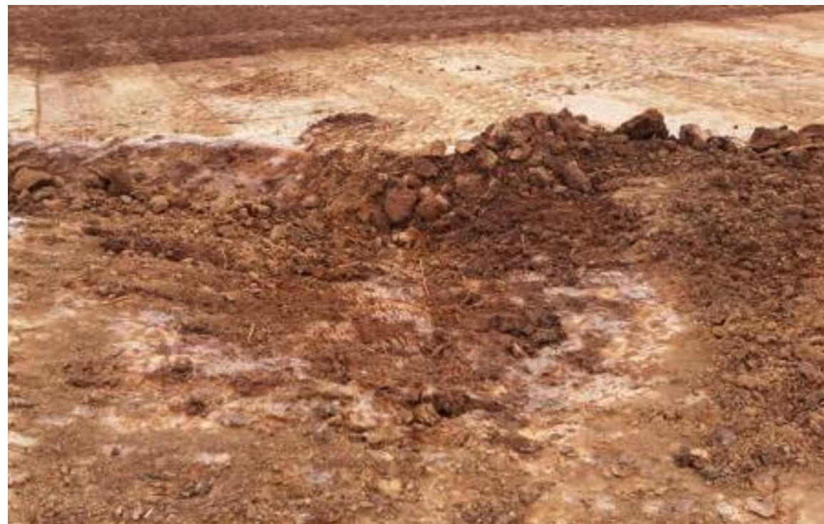
Removed tree root – D6 (west-south-west)
