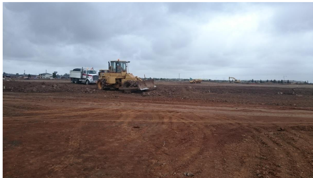
Compactor on Layer 2 in grid D4 (North) E4 (North) and F4 (North)
