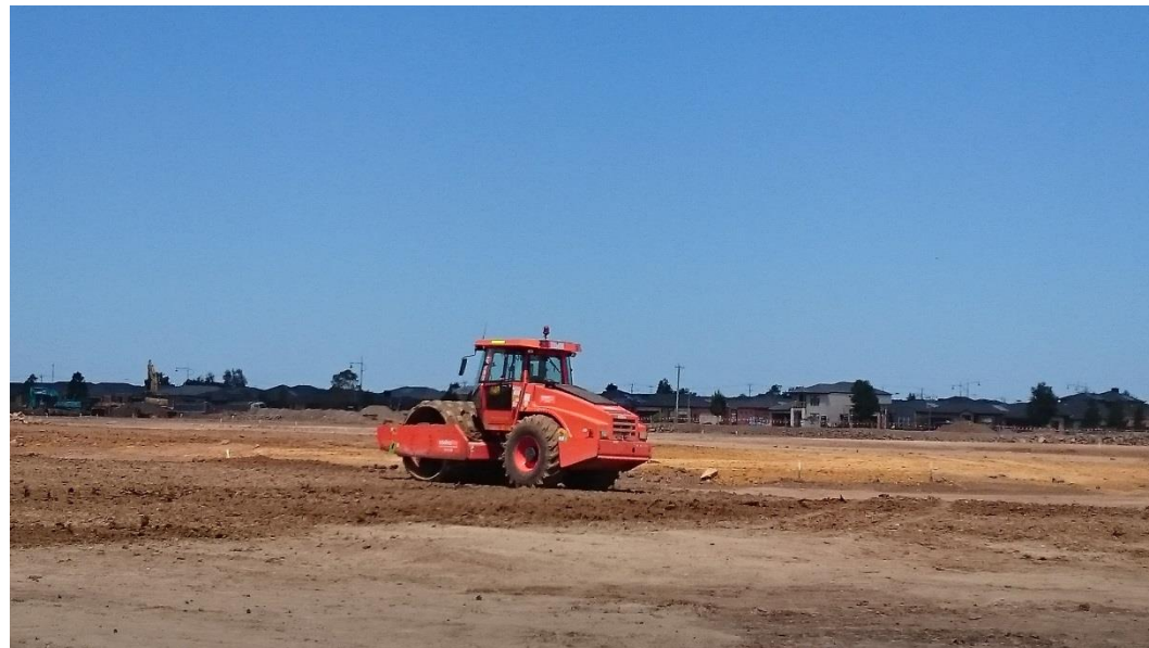
Pad foot roller and water cart on layer 2 in grid C5, C6, D5, D6
