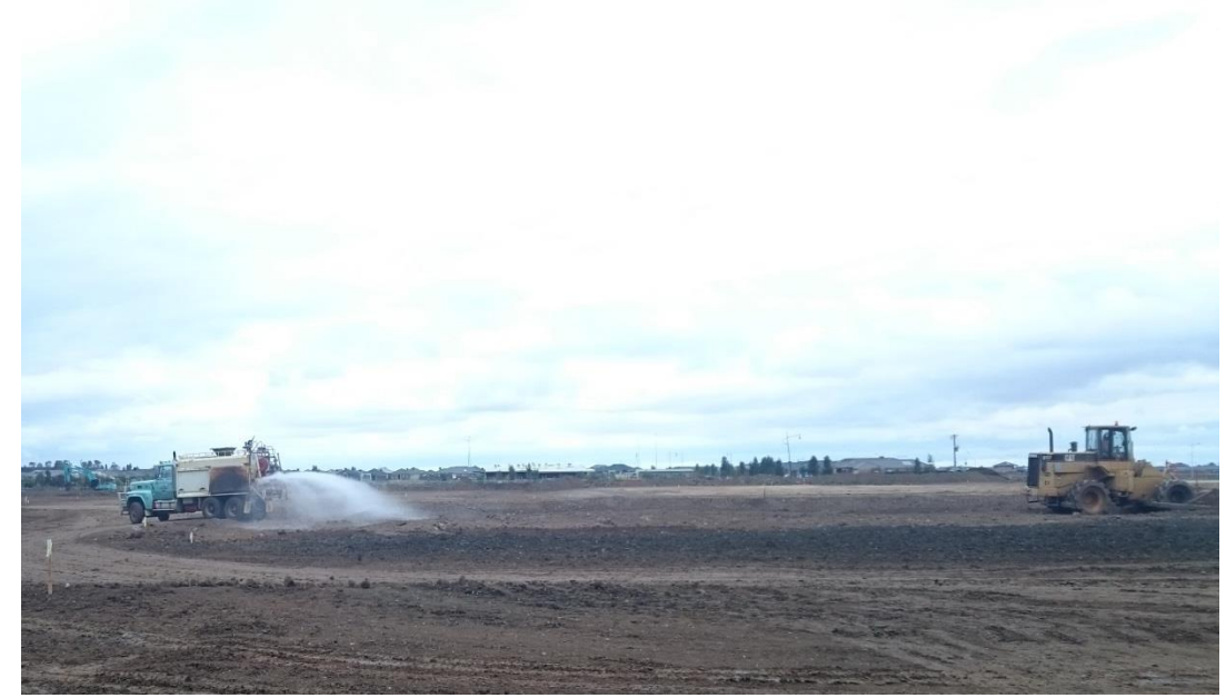
Compactor and water cart levelling fill and moisture conditioning layer 3 in grid A4, B4, C4, A5, B5, C5
