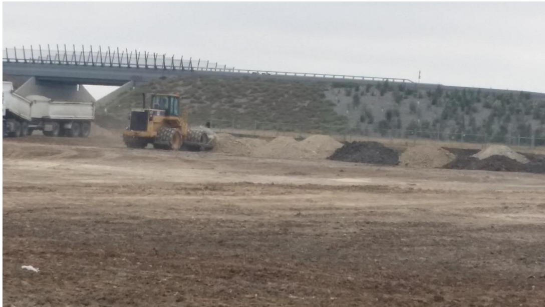
Stage 4: Placement and compaction of layer 1 material in grid N4 and N5.
