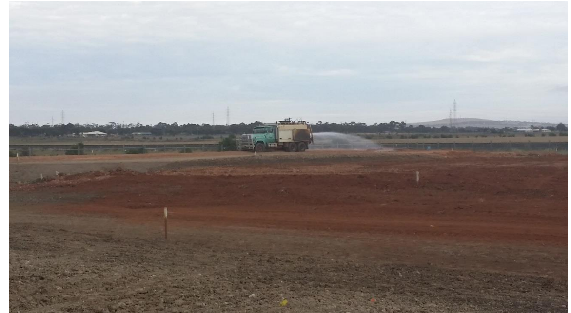
Stage 3: Moisture conditioning of excess placed material prior to grading in grid A5 (N) and A6
