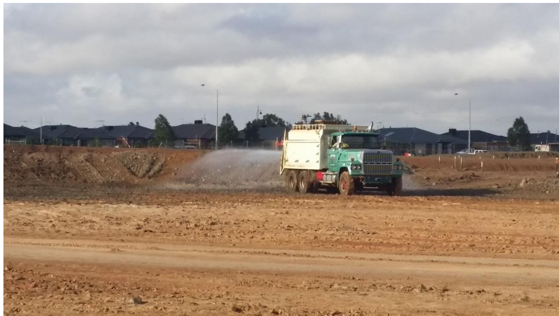
Stage 4: Moisture conditioning of placed layer 1 material in grid N2 (E) and O2.
