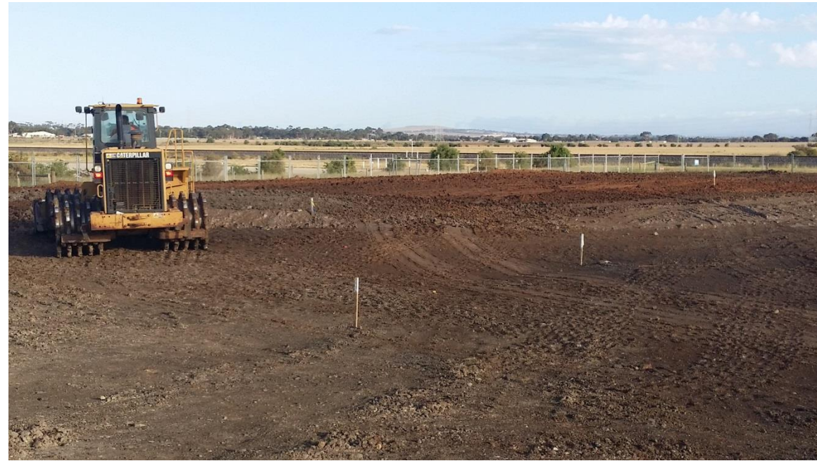
Stage 3: Compactor working newly placed layer 4 in grid A5 (N) and A6 (S)
