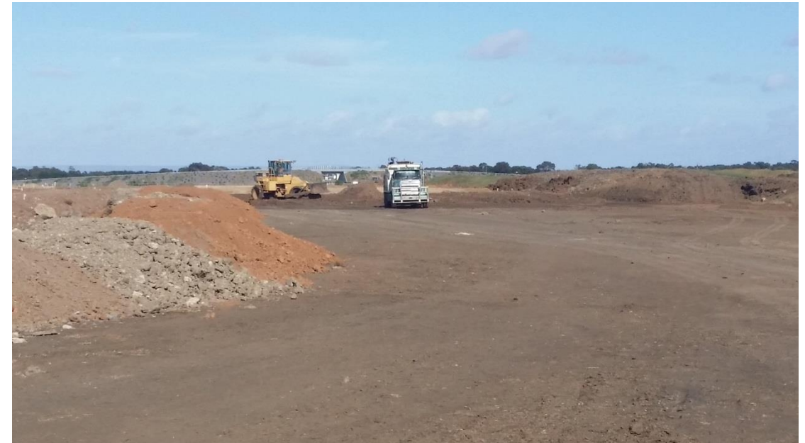
Stage 4: Placement of layer 1 silty clay fill, compacted and moisture conditioned in grid H5 (NE), H6 (SE), I5 (N), I6 (S), J5 and J6 (S).
