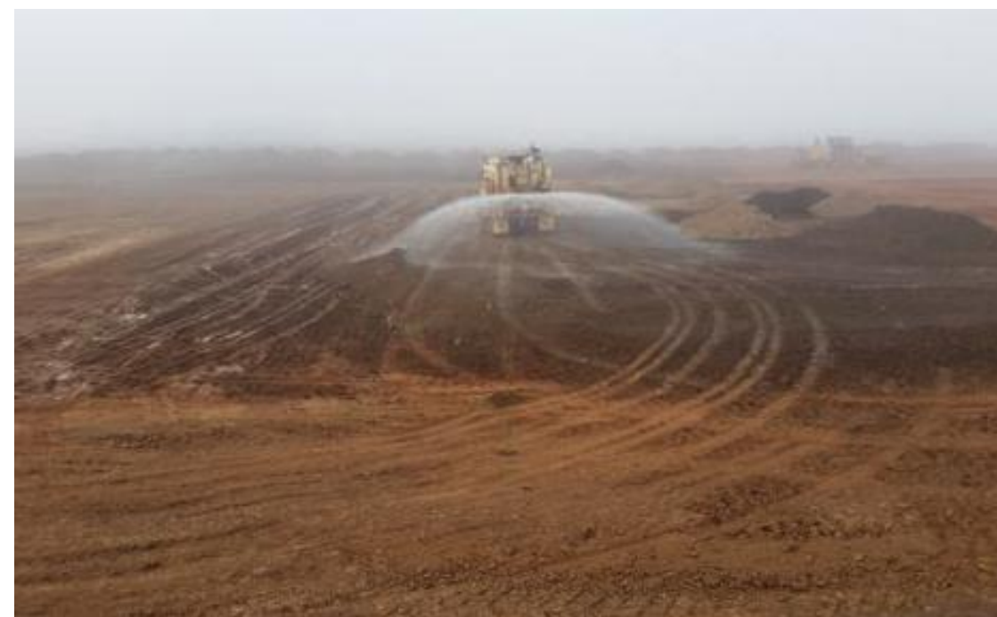
Water Cart moisture conditioning subgrade prior to placement of layer 1- G5 (north-west)/G6 (south-west).
