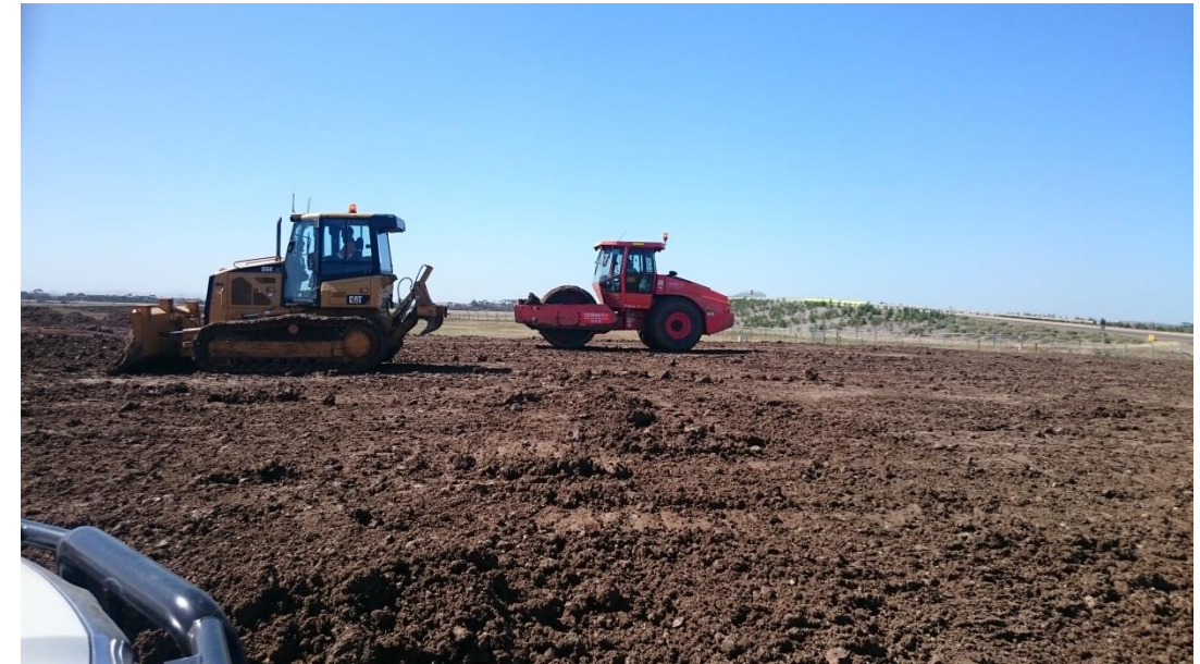
Stage 1: pad foot roller used on layer 7 in grid O1 (North) and O2 (South)
