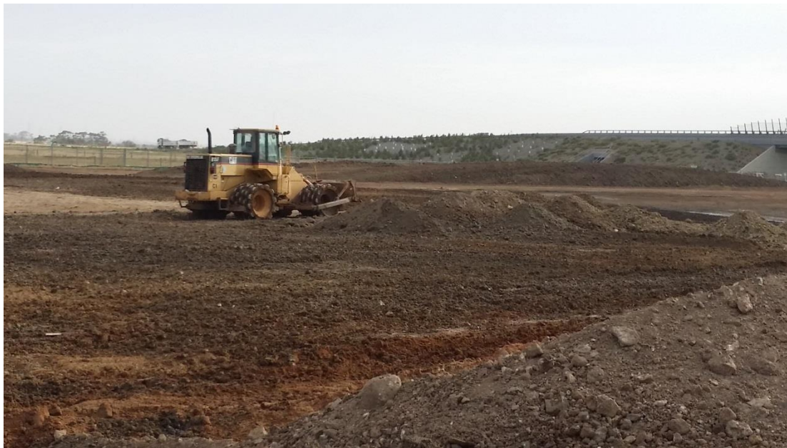
Stage 4: Placement and compaction of layer 1 material in grid L4, M4 and M5
