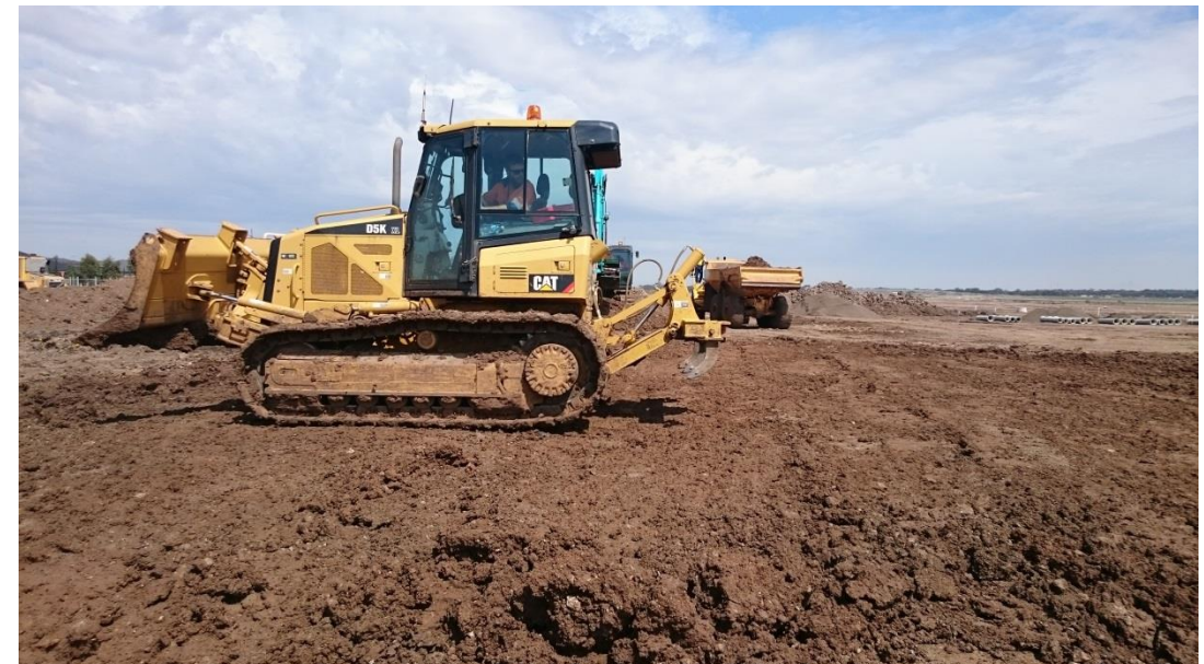
Stage 1: dozer placing material as part of layer 6 in grid M1 and M2
