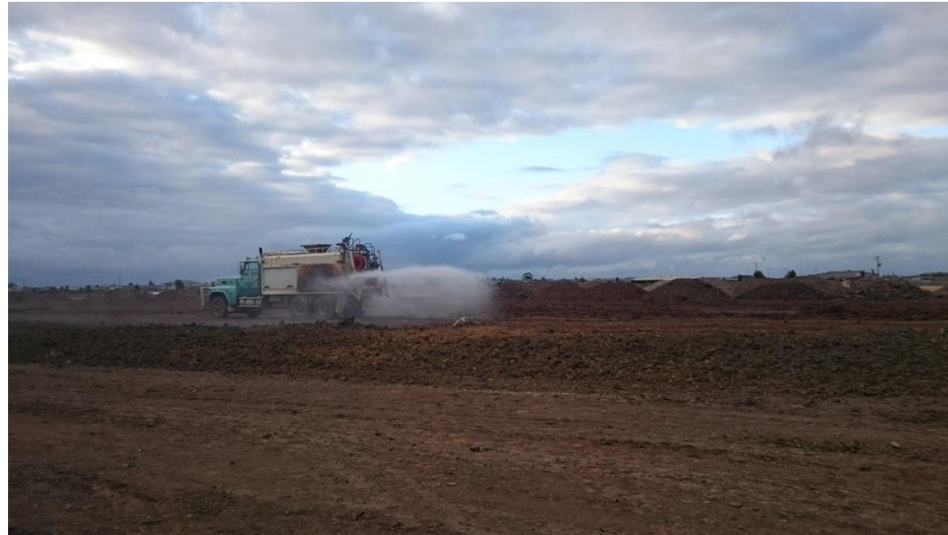
Water cart moisture conditioning layer 4 in grid A4, B4, C4 and A5, B5 and C5
