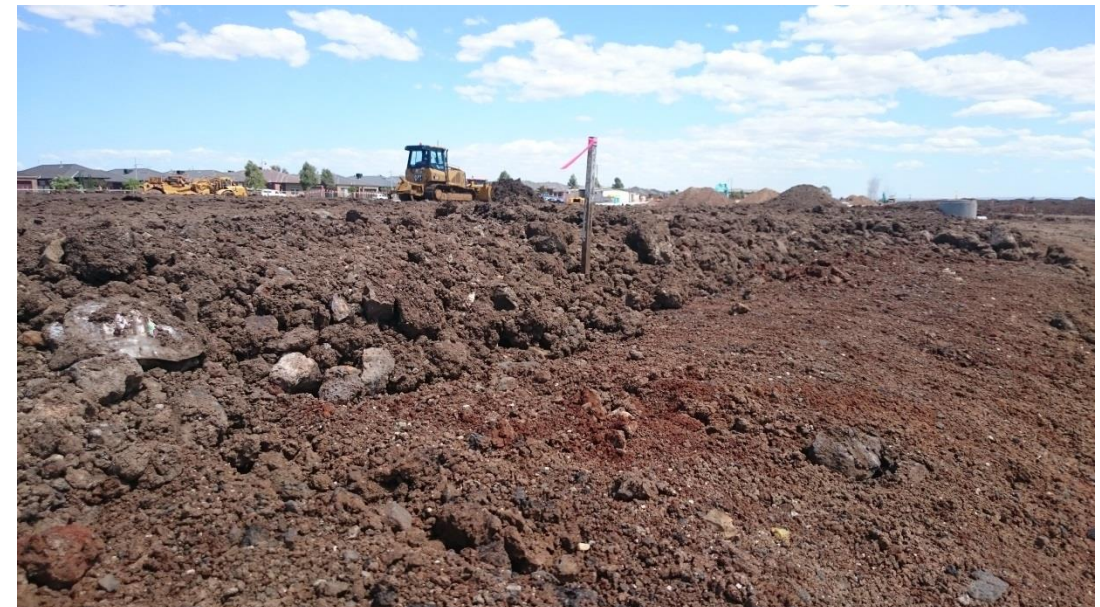
Stage 1-Layer 7 thickness: dozer pushing more material as part of layer 7 in grid N1 (North East) and N2 (South East).
