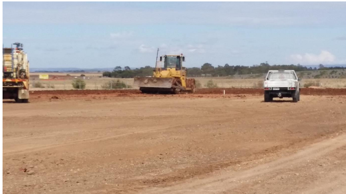
Stage 3: Compacting of scarified and moisture conditioned material in grid B5, B6, C5 (W) and C6 (W).
