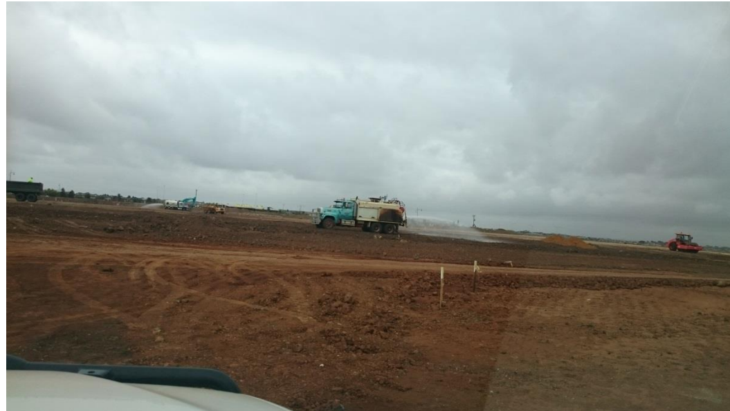
Water cart moisture conditioning layer 2 in grid D4 (North) E4 (North) and F4 (North)
