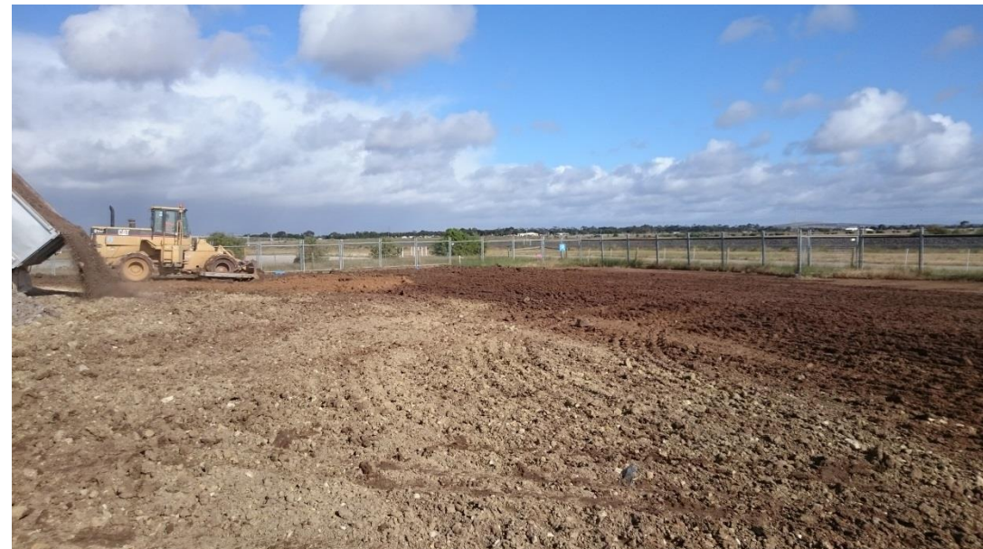
Stage 4: compactor placing layer 1 upon subgrade in the northern most side of Stage 3 (refer to Stage 3 site plan)
