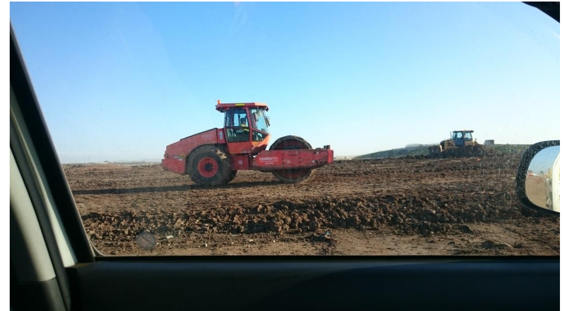
Stage 1: pad foot roller used on layer 7 in grid O1 (North) and O2 (South)
