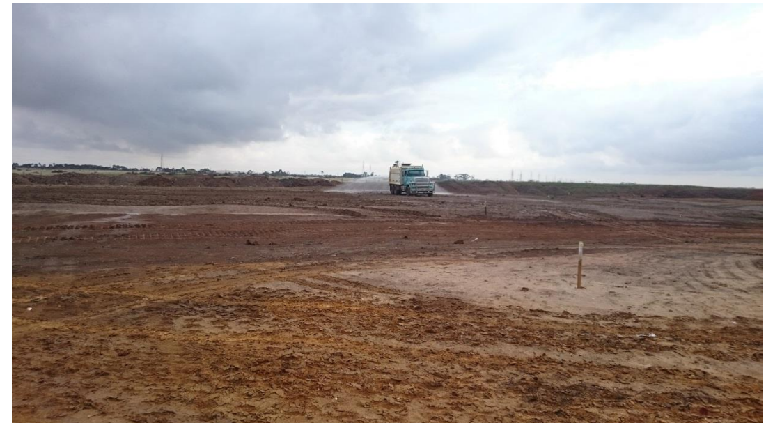
Stage 3: water cart being used on layer 3 in grid D5 and D6 prior to placement of fill
