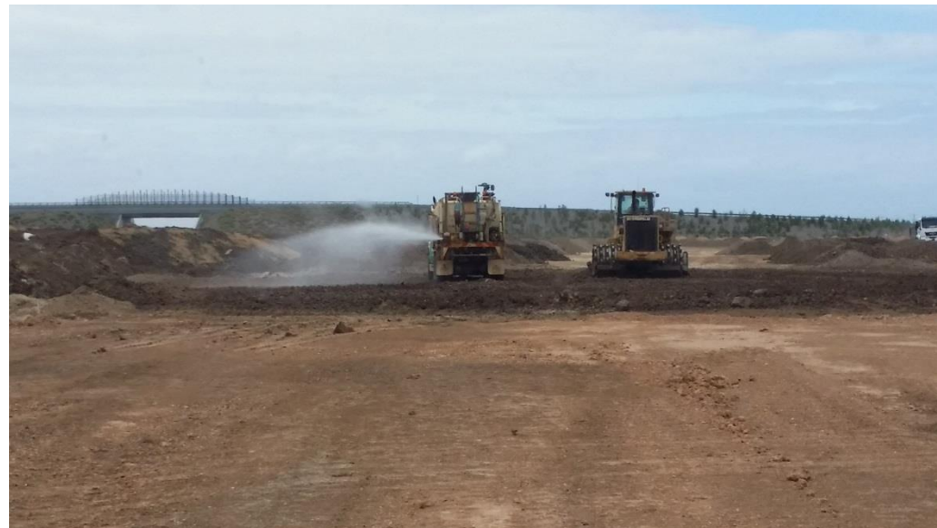
Stage 4: Moisture conditioning of layer 2 material after placement in grid H5 (NE), H6 (SE), I5 (N) and I6 (S)
