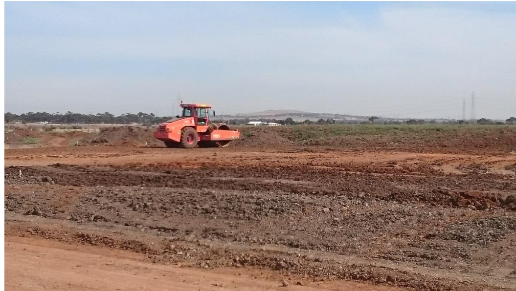
Pad foot roller on layer 2 in grid F5, F6, G5 and G6
