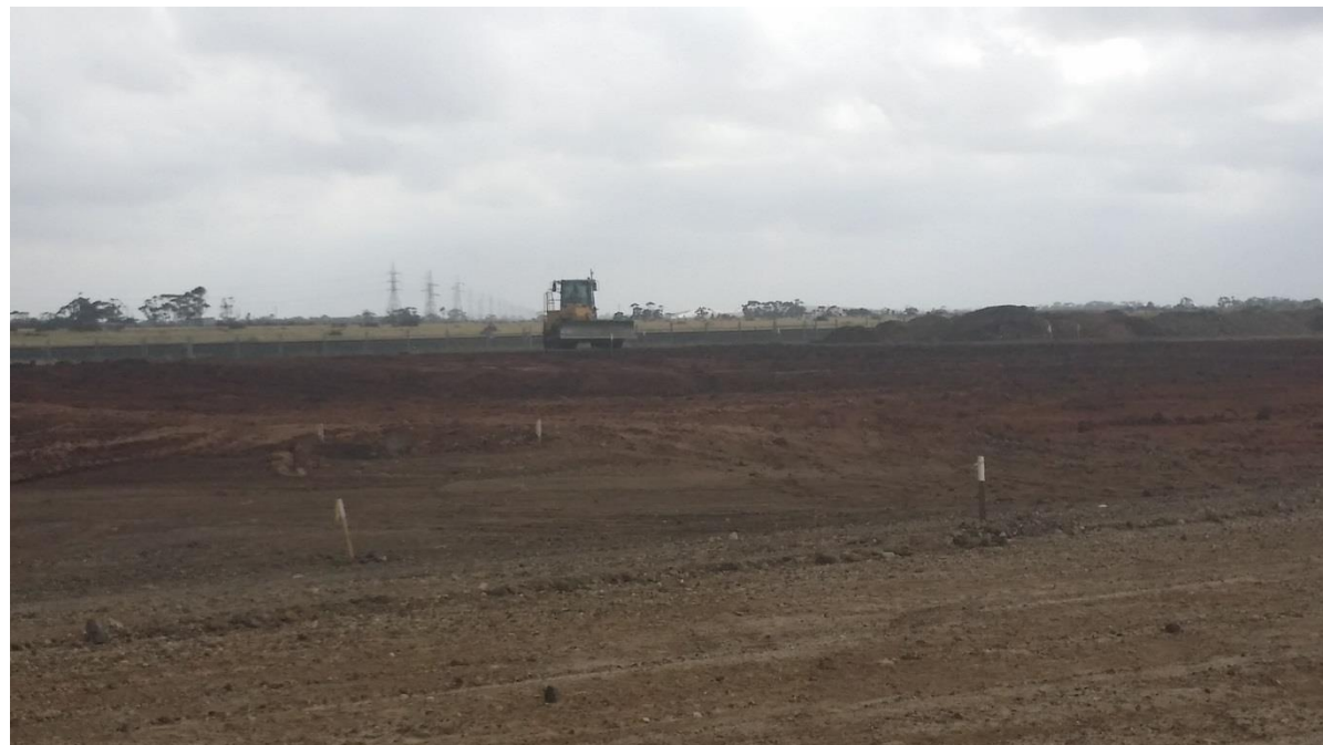
Stage 3: Compacting of scarified and moisture conditioned material in grid B5, B6, C5 (W) and C6 (W).
