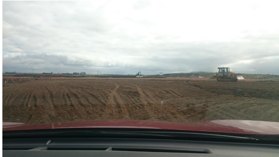
Stage 1: placement of topsoil in in grid O1, O2, N1 and N2
