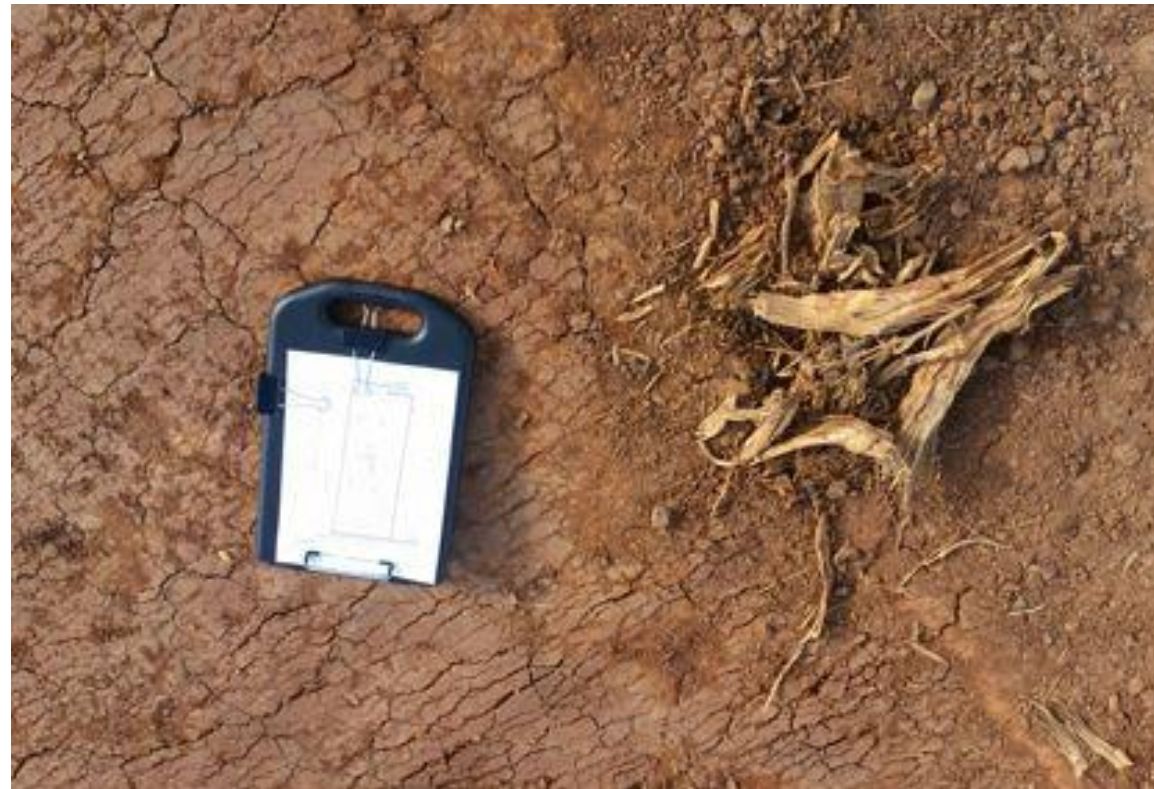
Tree root within subgrade – D6 (south-south-west)
