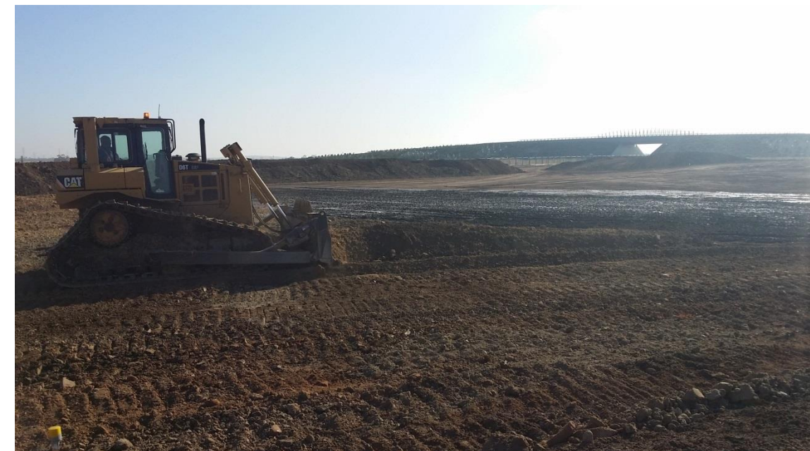
Stage 4: Placement of material by large dozer in grid K5 and K6 (S)
