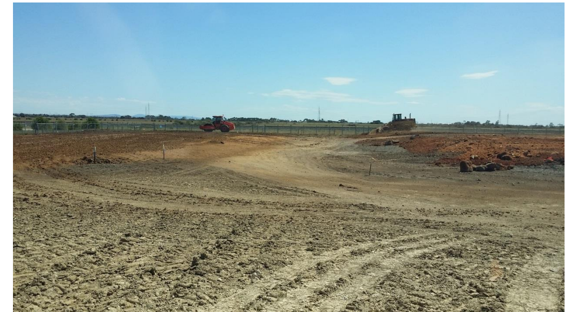
Stage 3: Layer 1 being compacted and rolled in grid A6 (N) and A7 (S)
