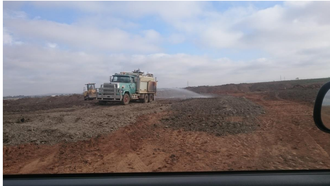
Compactor and Water cart moisture conditioning layer 2 in grid E5 and E6
