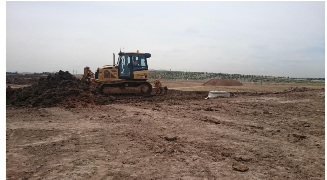
Stage 1: dozer placing material on layer 6 in grid O2 (East) in L-Shape
