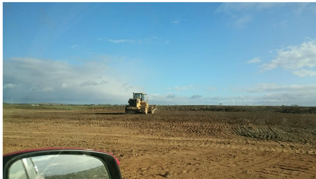
Stage 3: layer 3 in grid G5 (W) and G6 (W) being compacted prior to bring rolled and tested
