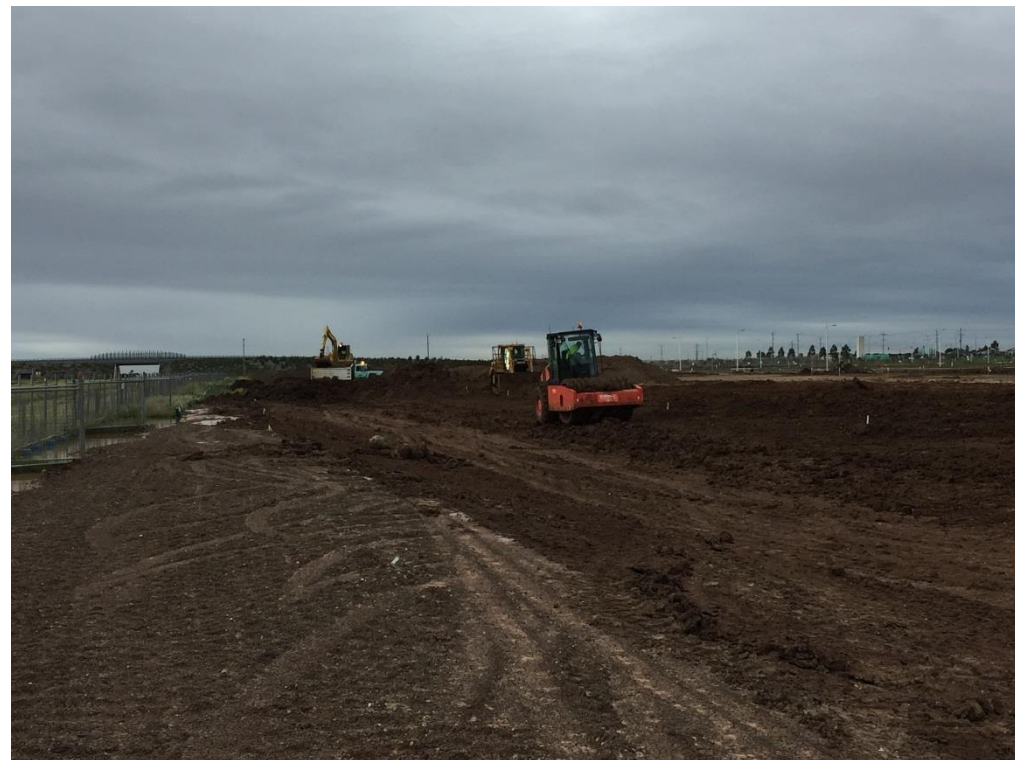
Stage 3: Pad-foot roller rolling newly placed Layer 2 in grid sections E6, F6, G6
