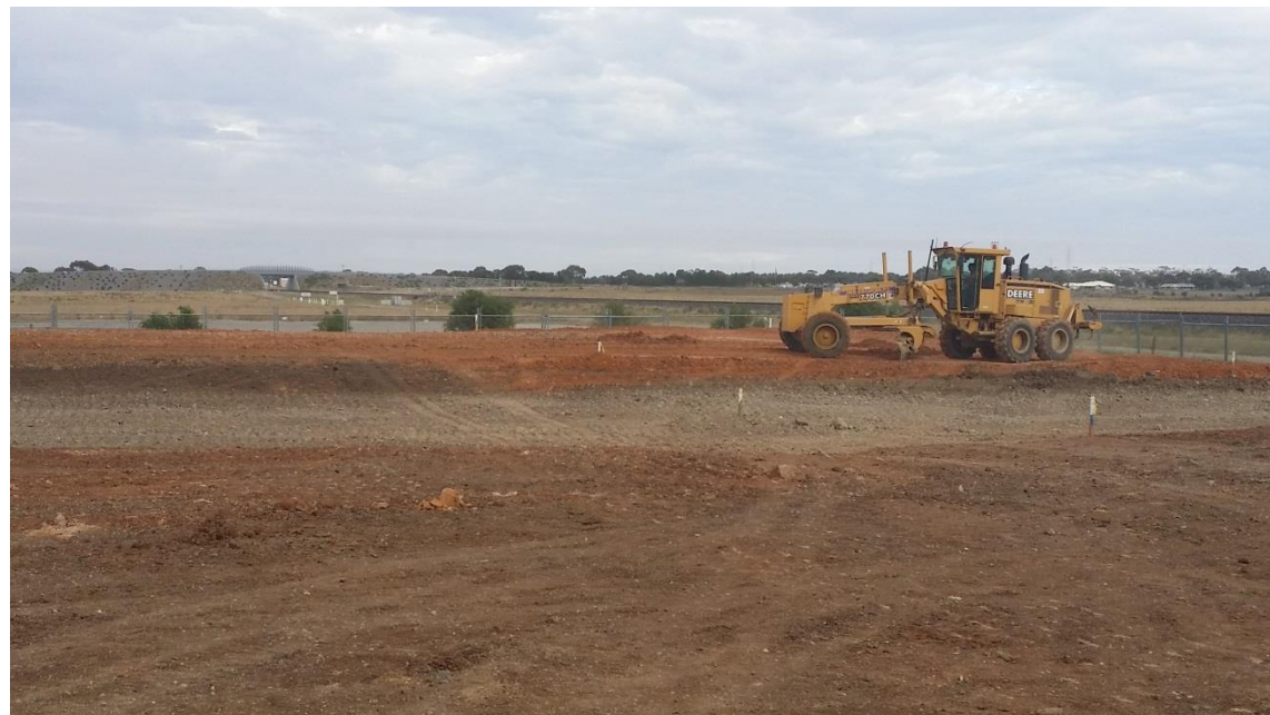
Stage 3: Grading of excess placed material in grid A5 (N) and A6
