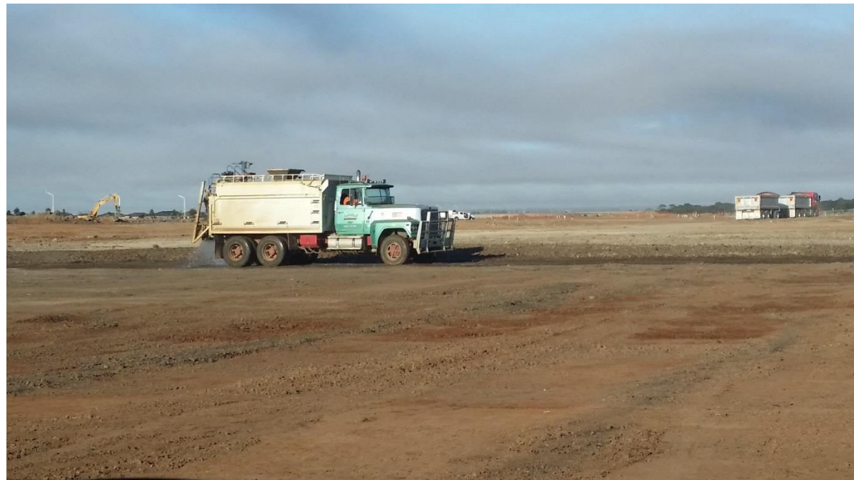
Stage 4: Moisture conditioning of subgrade pre placement of layer 1 material in grid N4 and N5
