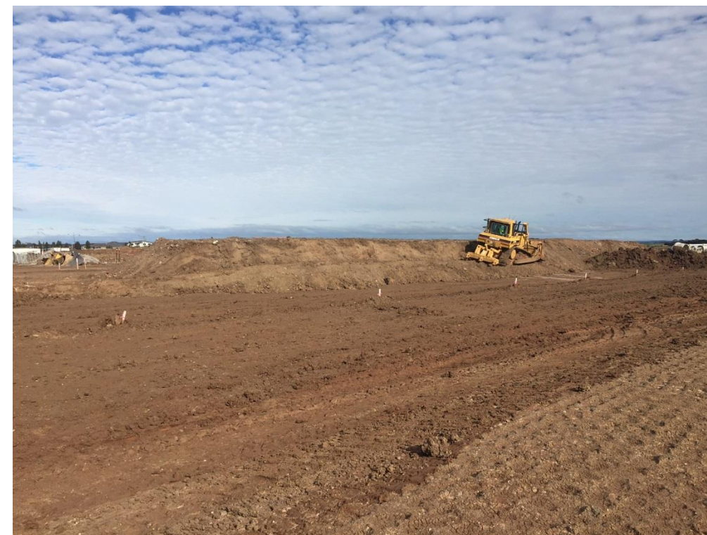
Stage 3: Bull Dozer pushing fill stockpile in grid sections B6, C6 & D6 as Layer 2
