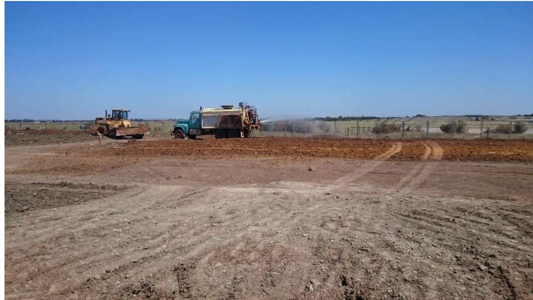
Compactor and Water cart moisture conditioning layer 2 in grid A5 and A6
