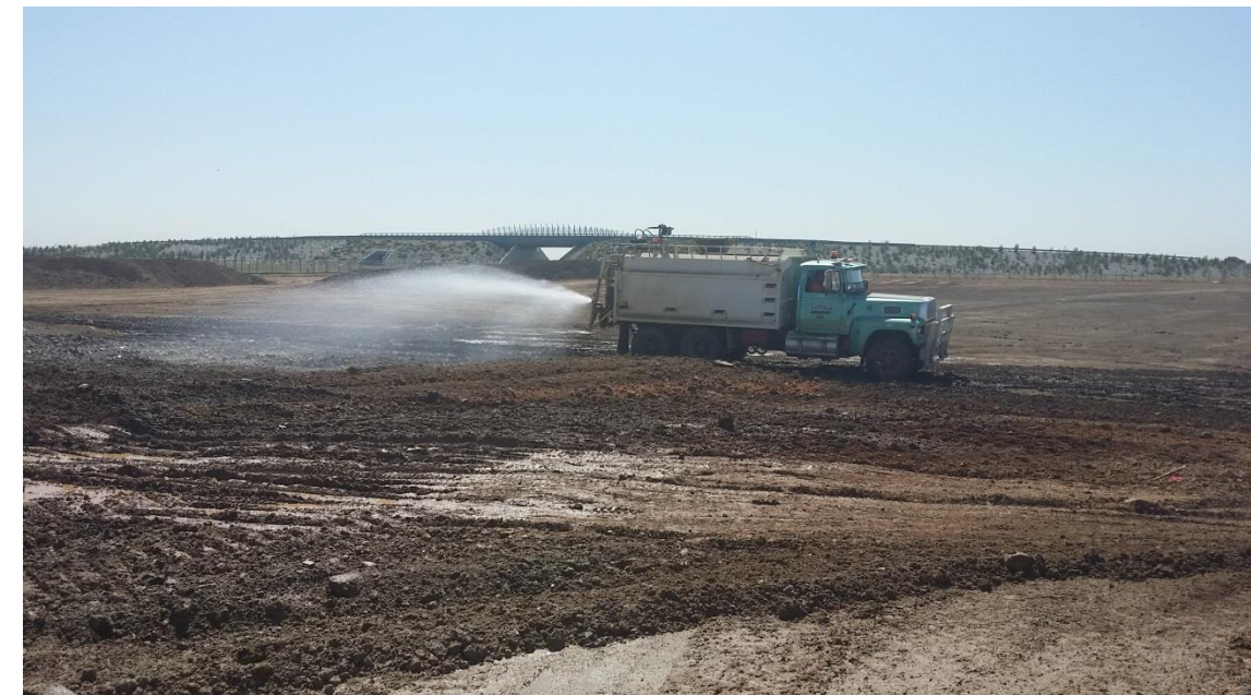
Stage 4: moisture conditioning of layer 1 material in grid J5, J6 (S), K5, K6 (S), L4, L5 and L6 (SE)
