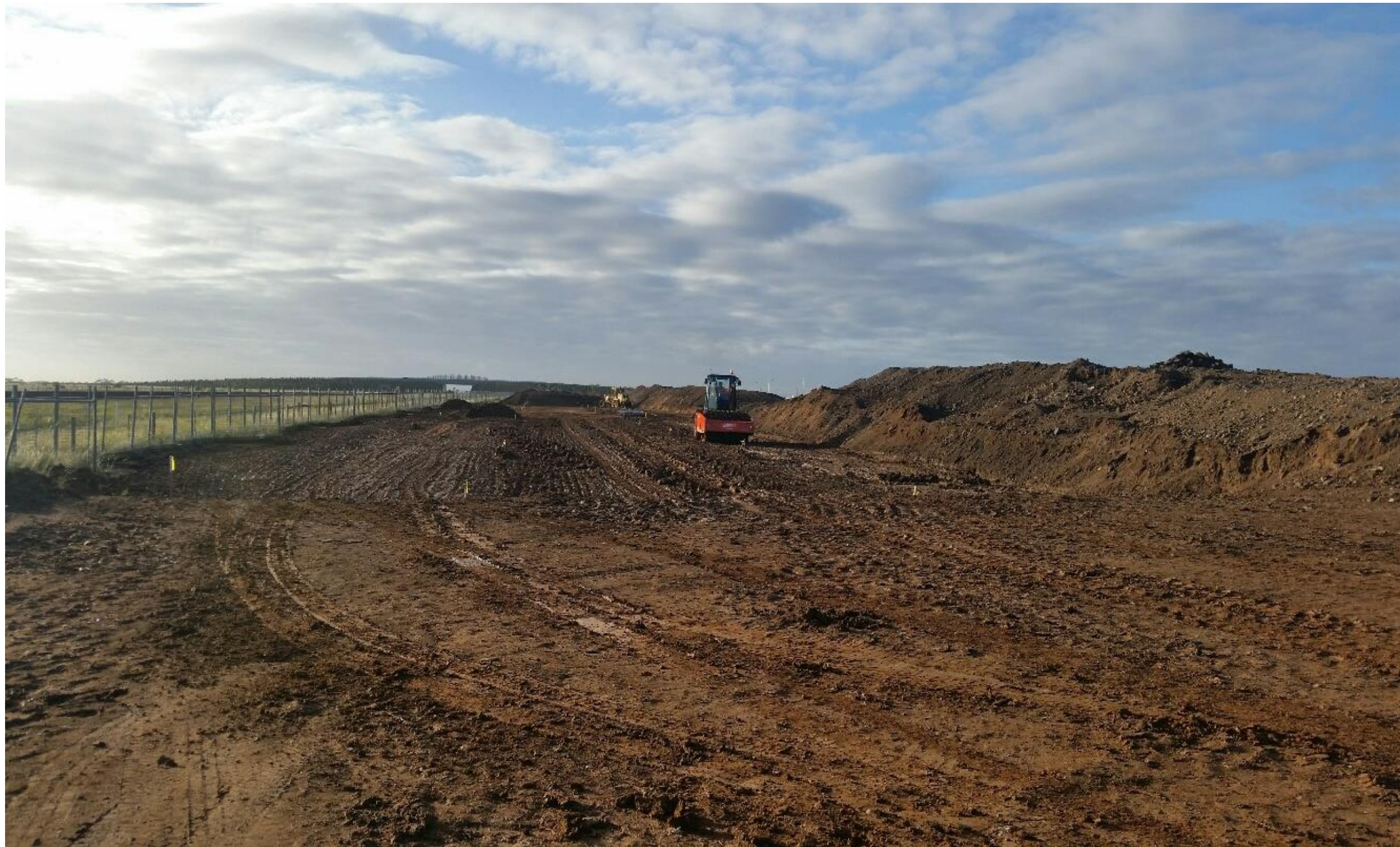
3. General view of the site and Pad foot roller working on layer 1 due to failed test
