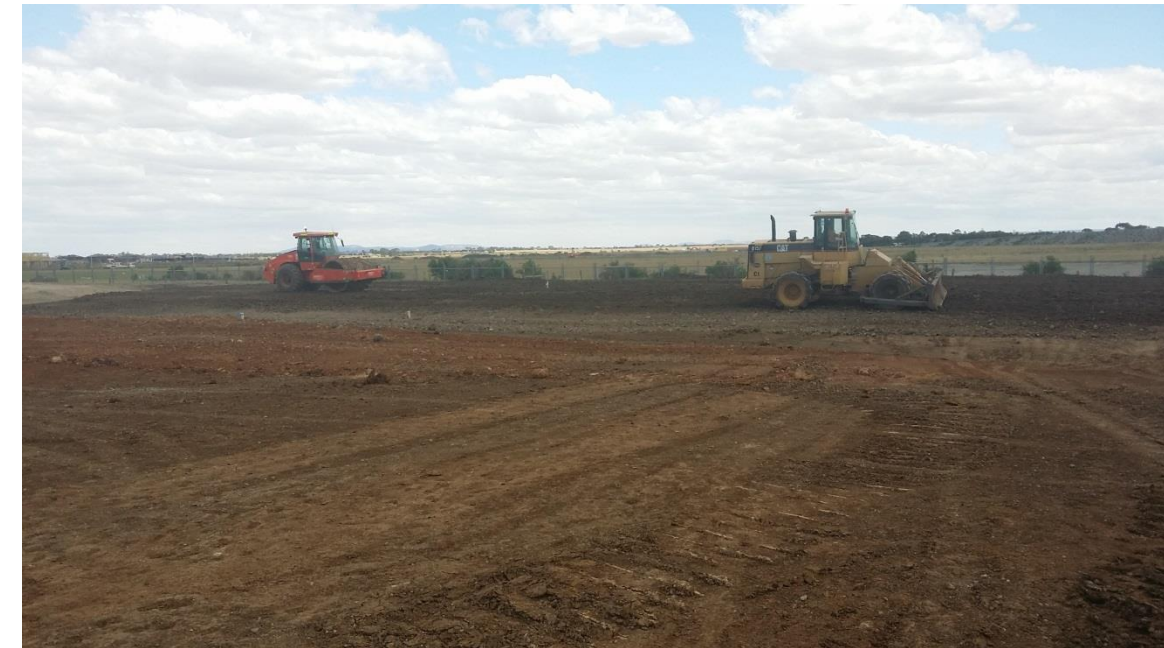
Stage 3: Layer 4 in grid A5 (N) and A6 (S) and layer 2 in grid A6 (S) being compacted and rolled
