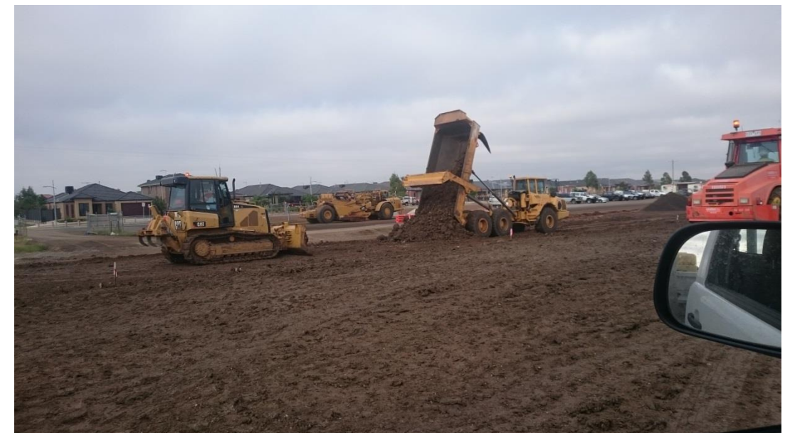
Stage 1: dozer pushing more silty clay fill as part of layer 6 along road D in grid O1 (centre) and N1 (East)
