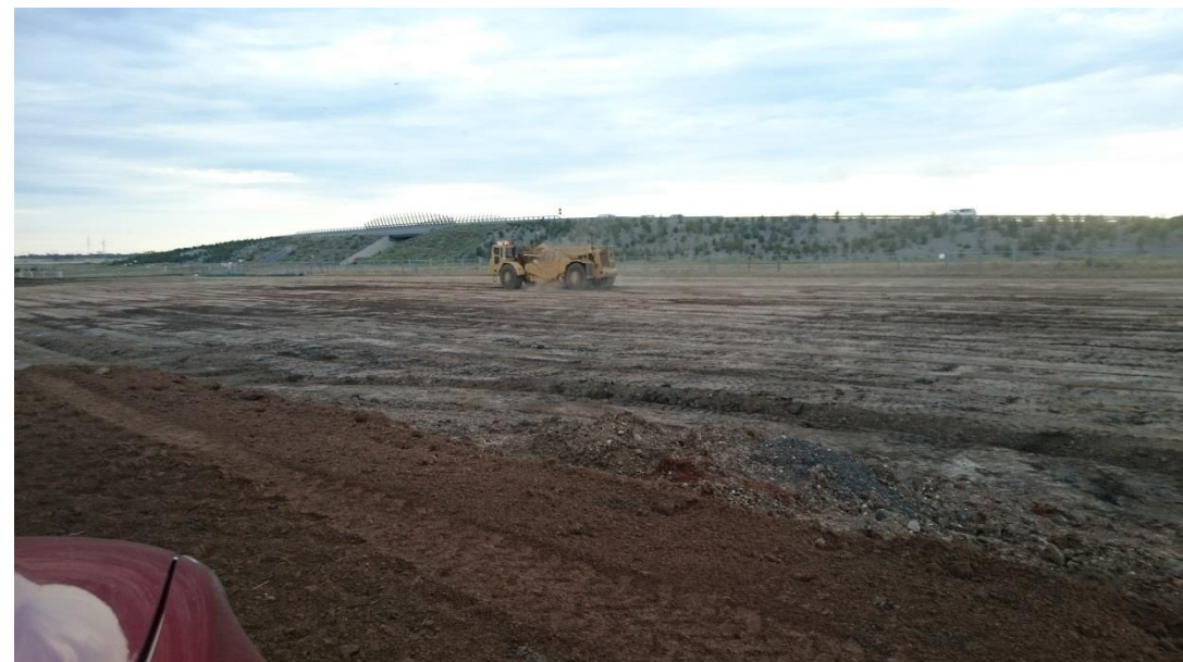
Stage 4: scraper removing topsoil layer as shown in Stage 4 site plan above
