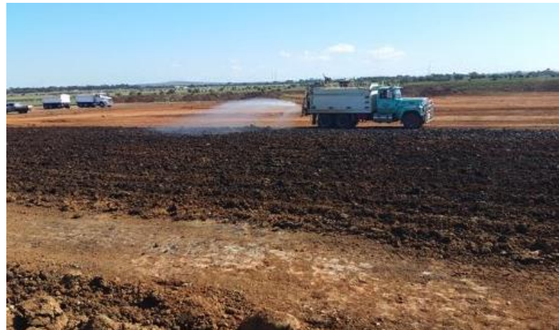
Water Cart moisture conditioning layer 1 – E4 (north-north-east), F4 (north-north-east), and G4 (west-north-west).
