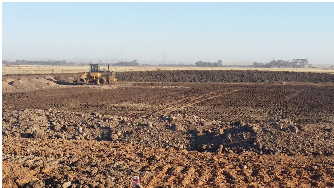
Stage 4: Placement and compaction of layer 1 material in grid N4, N5, O4 and O5.
