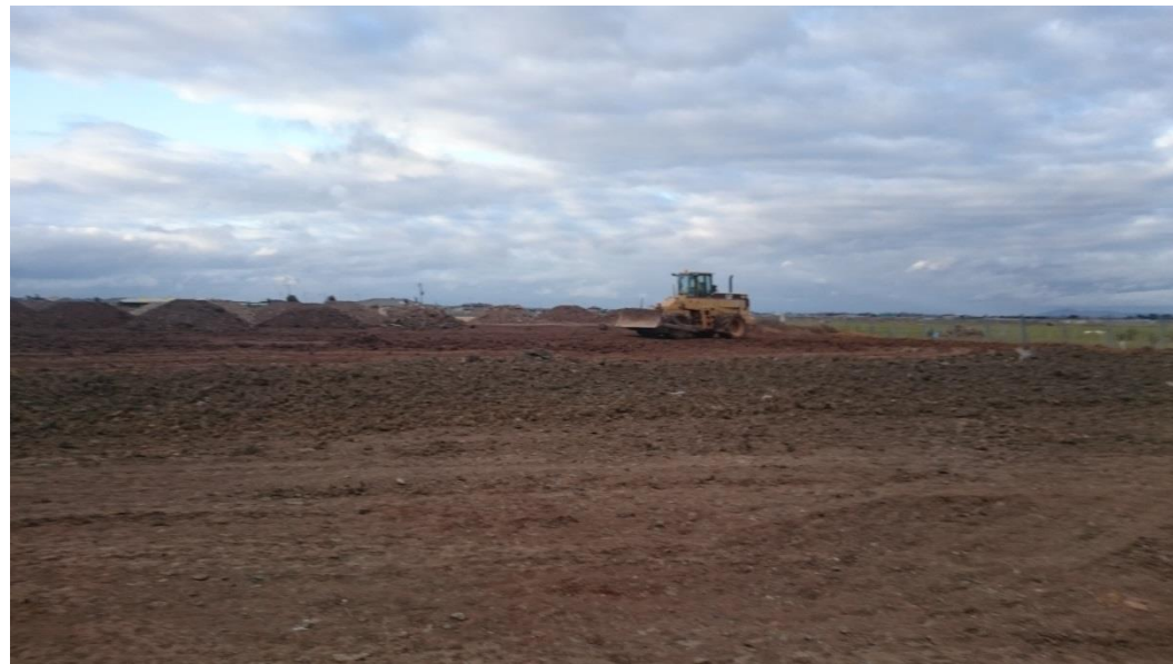
Compactor on layer 4 in grid A4, B4, C4 and A5, B5 and C5
