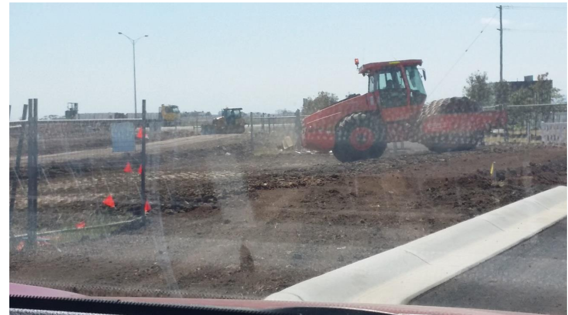
Stage 1 & 4: Placement and rolling of road fill material in grid O1, P1 and P2
