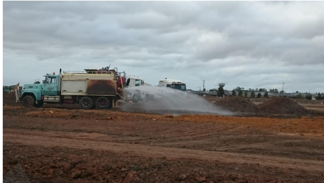
Water cart moisture conditioning layer 2 in grid D4, E4, F4 and G4
