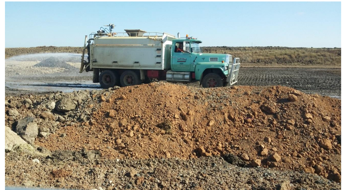
Stage 4: moisture conditioning of layer 1 material in grid J5, J6 (S), K5 and K6 (S)
