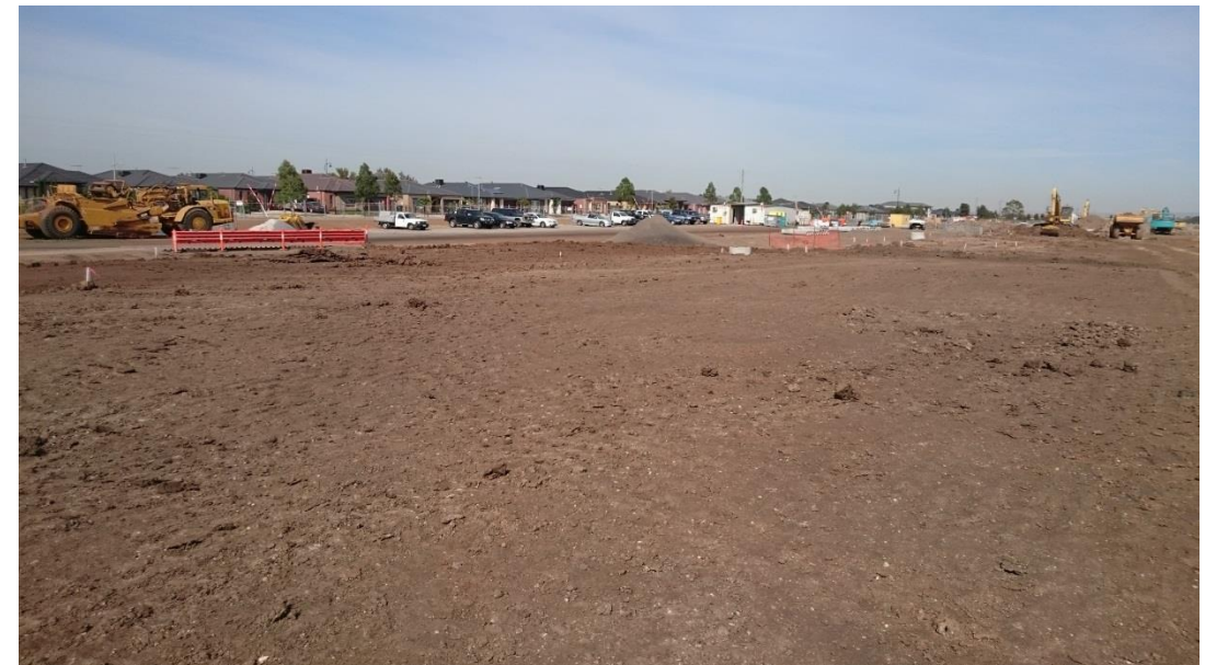
Stage 1: View of layer 7 placed in grid O1, O2 and layer 6 along road D in grid O1 (centre) and N1 (East)
