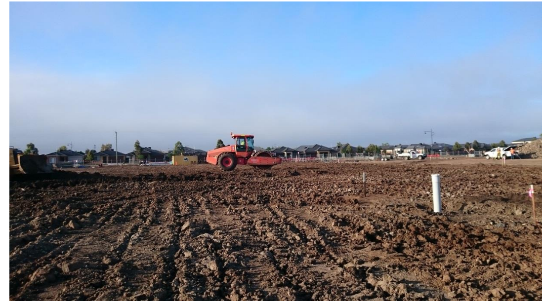
Stage 1: pad foot roller being used on layer 6 in grid K1 and K2
