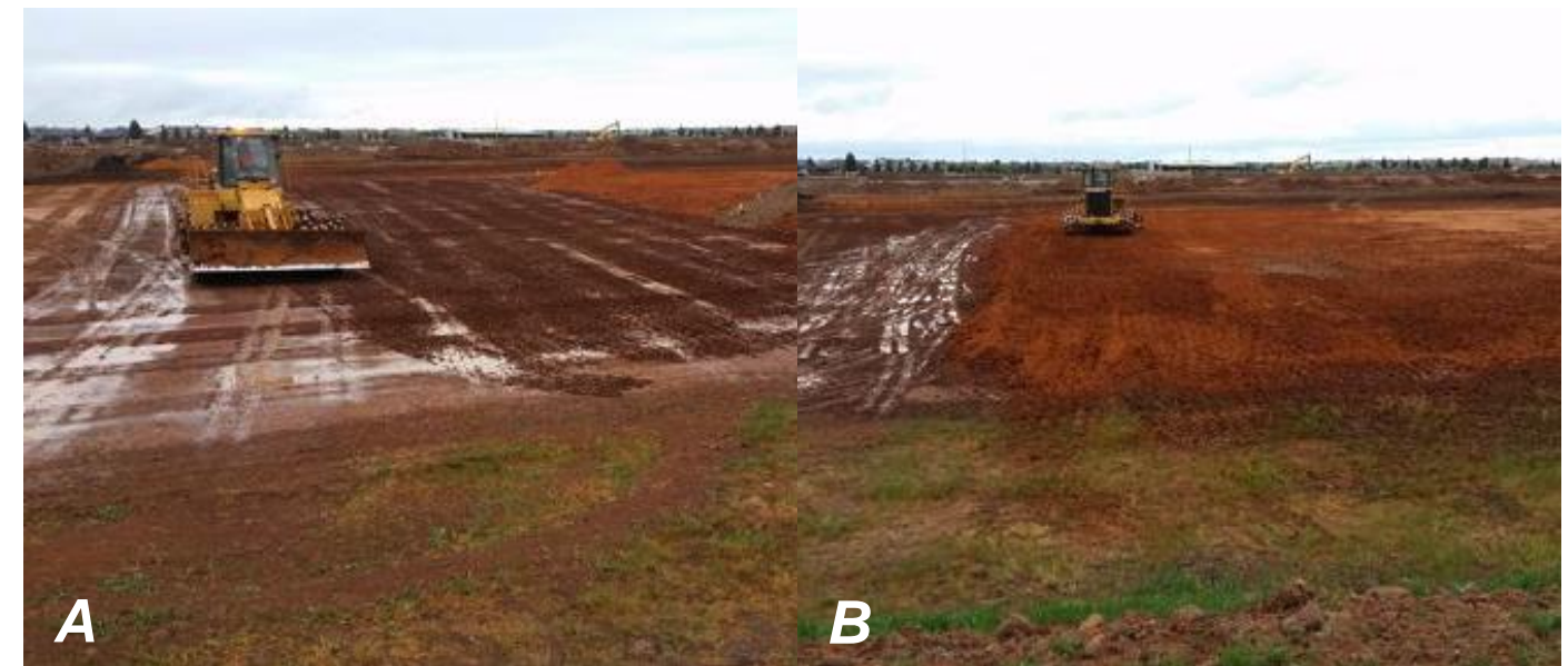
Compactor roughing up/compacting subgrade (A) and 100mm sublayer (B) - F6 (south), F5 (north-east) and F4 (north-east).
