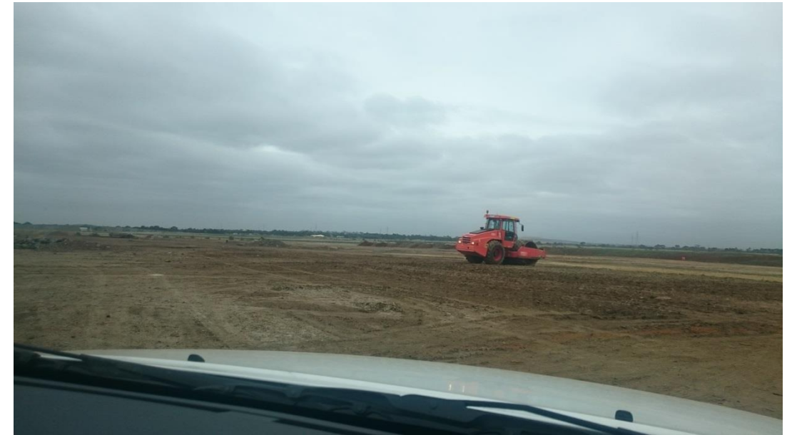
Stage 3: Pad foot roller being used to roll layer 3 and 4 (refer to Stage 3 site plan above)
