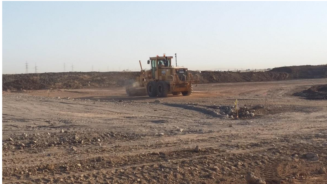
Stage 3: Spreading and grading of material on road K in grid H5 and H6
