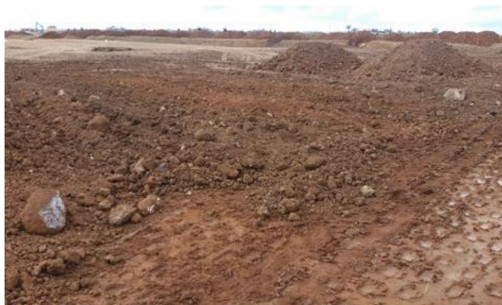
Some oversize boulders (>200mm 3 ) present in fill – Column A
