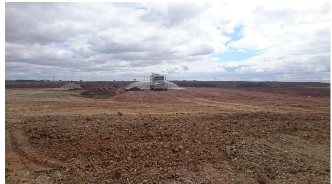
Stage 3: water cart being used on layer 3 in grid G5 and G6 prior to testing
