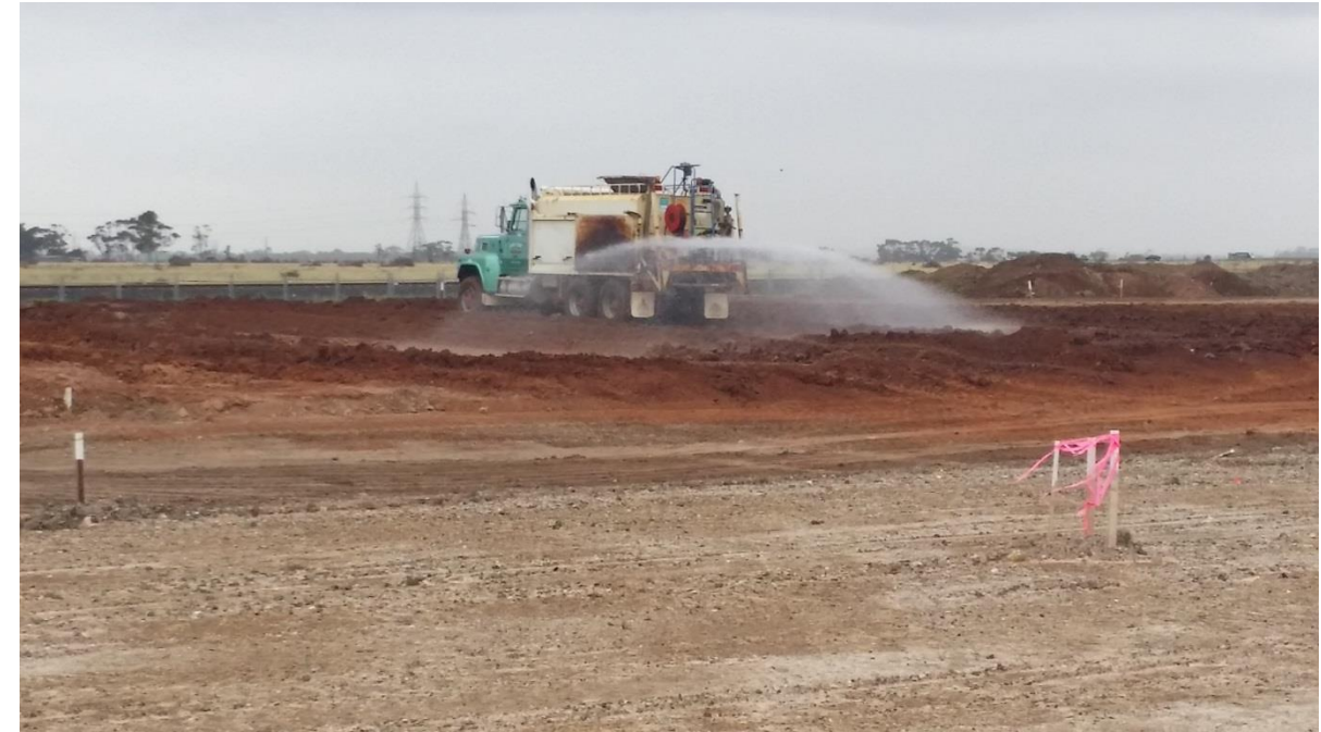
Stage 3: Moisture conditioning of scarified material in grid B5, B6, C5 (W) and C6 (W).
