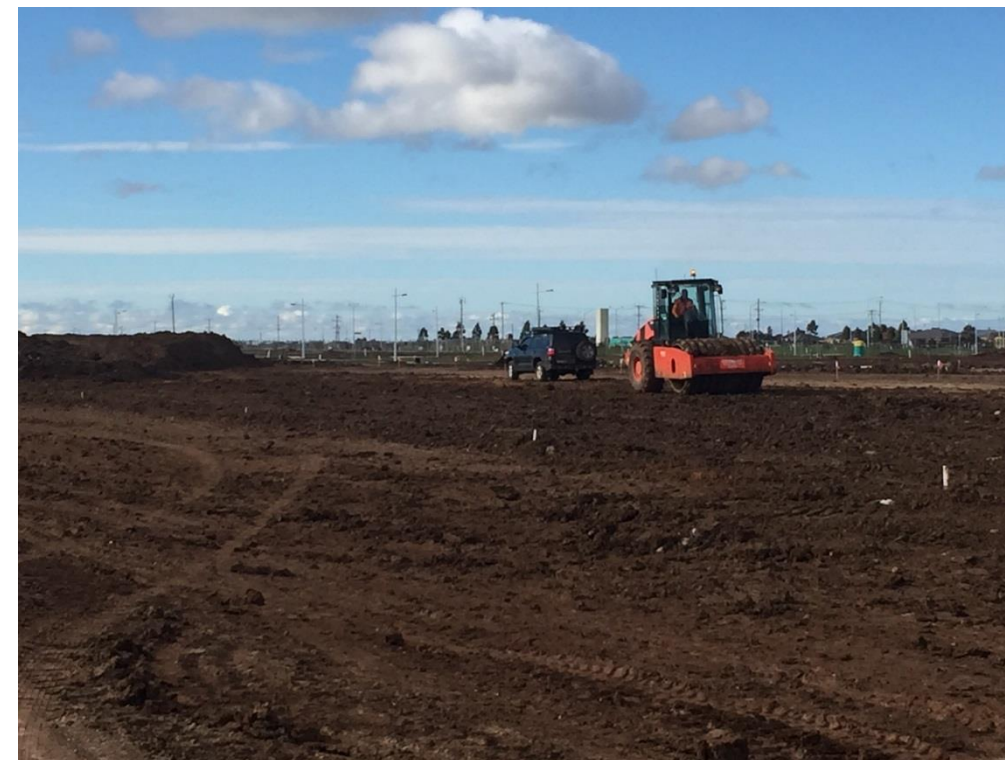
Stage 3: Pat-foot roller compacting newly placed layer 3 in grid sections E6, F6, G6
