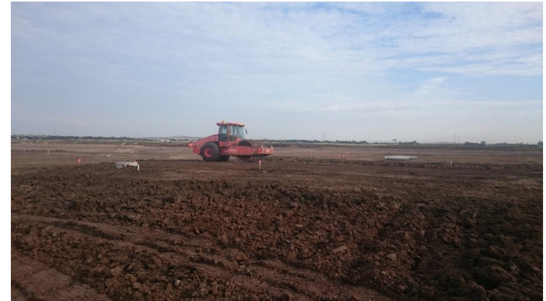
Stage 1: pad foot roller being used on layer 6 in grid J2 prior to testing
