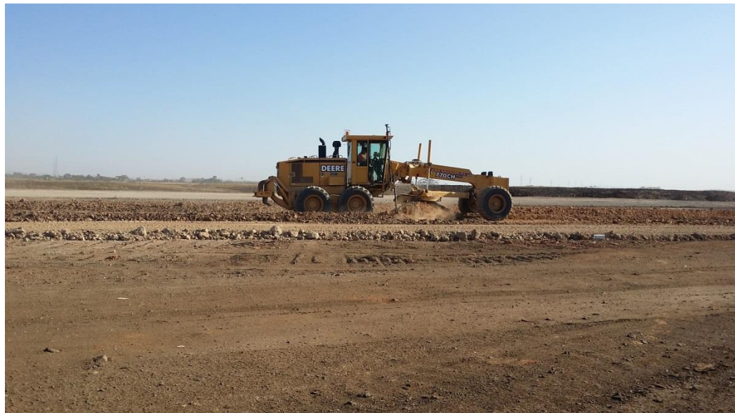
Stage 3: Spreading and grading of material in grid D4, E4, F4 and G4
