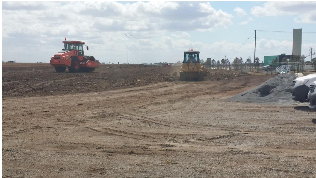
Stage 1: Small dozer placing fill on road D grid N1 and O1 which is then rolled by padfoot.
