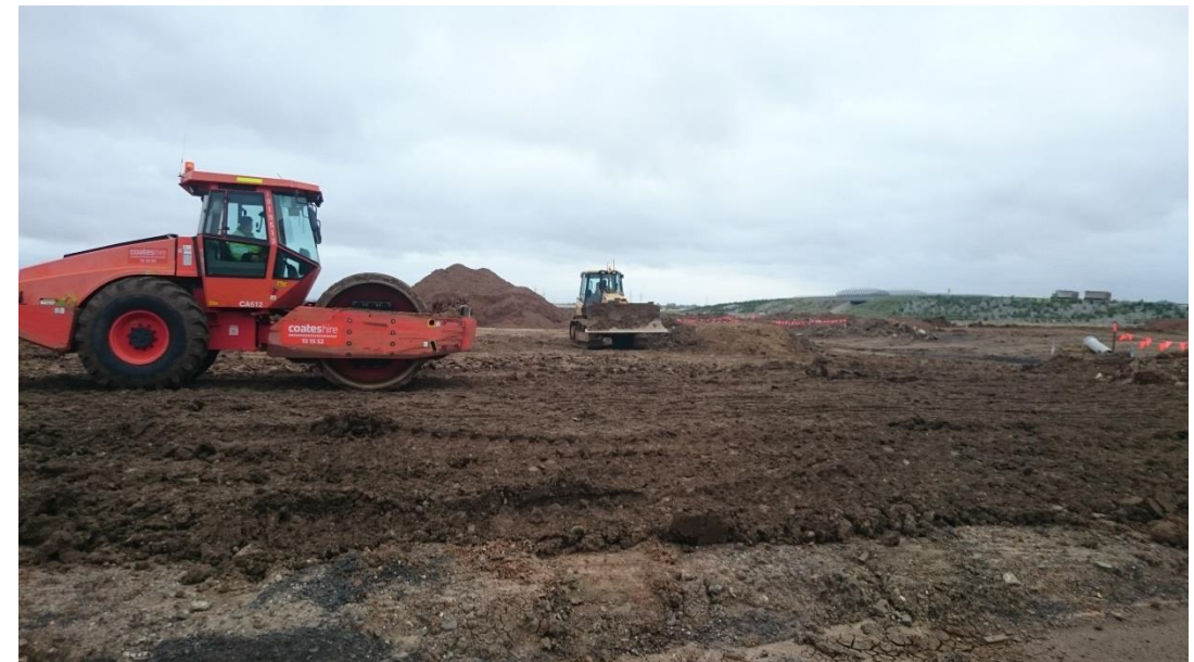
Stage 1: dozer placing material as part of layer 6 in grid M1 and M2
