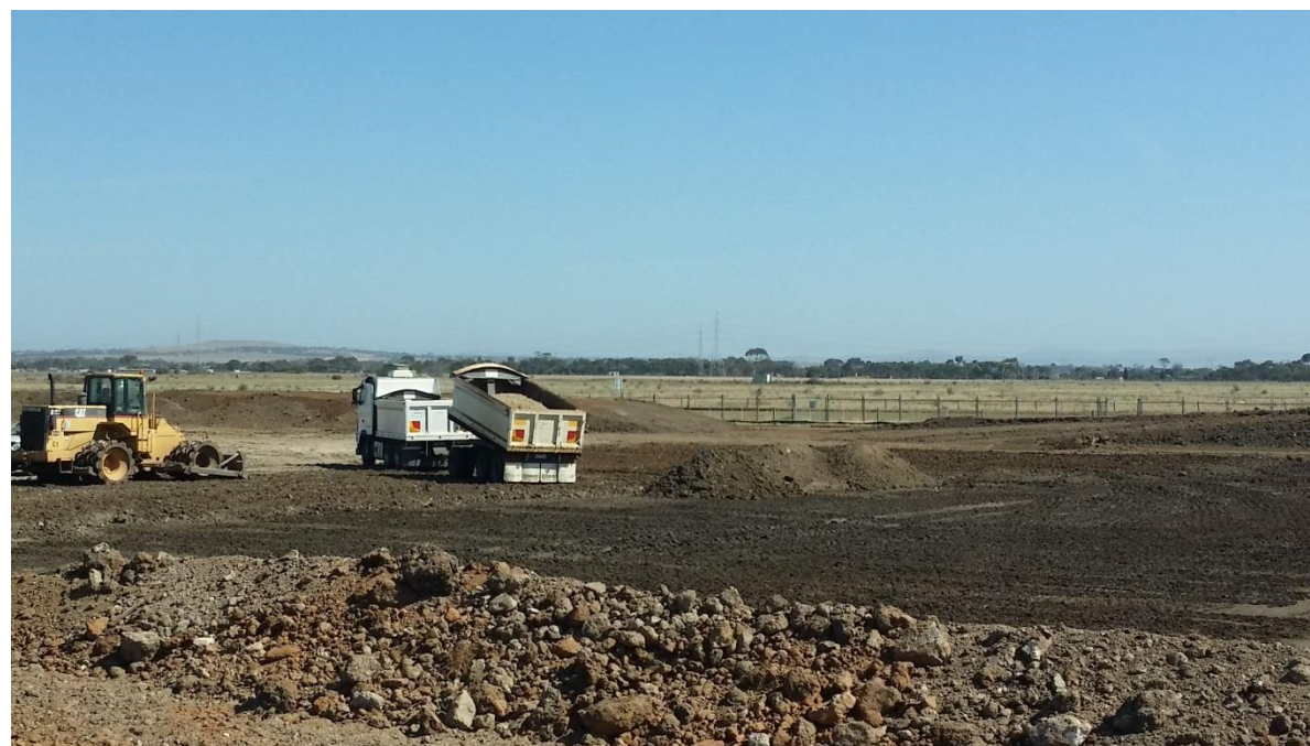
Stage 4: Placement and compaction of layer 1 material in grid N4 and N5
