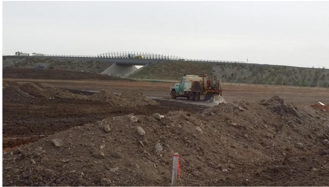
Stage 4: Moisture conditioning of subgrade pre placement of layer 1 material in grid N4 and N5
