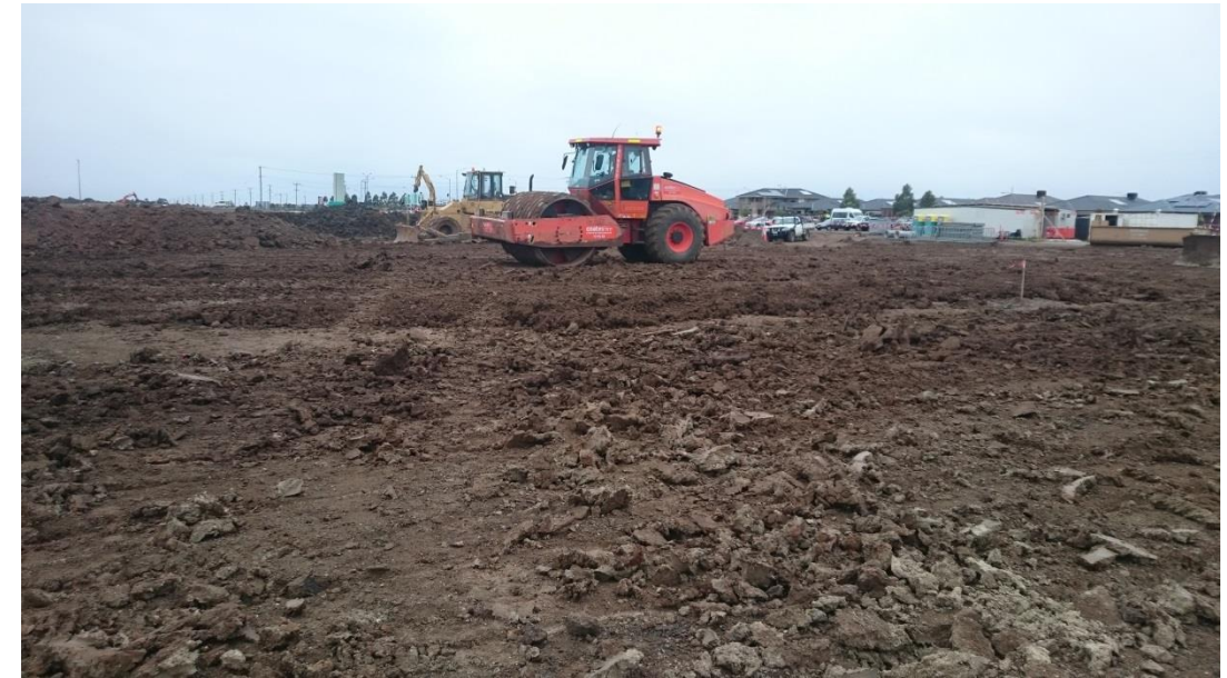
Stage 1: Pad foot roller being used to compact layer 6 in grid K1 and K2 prior to testing
