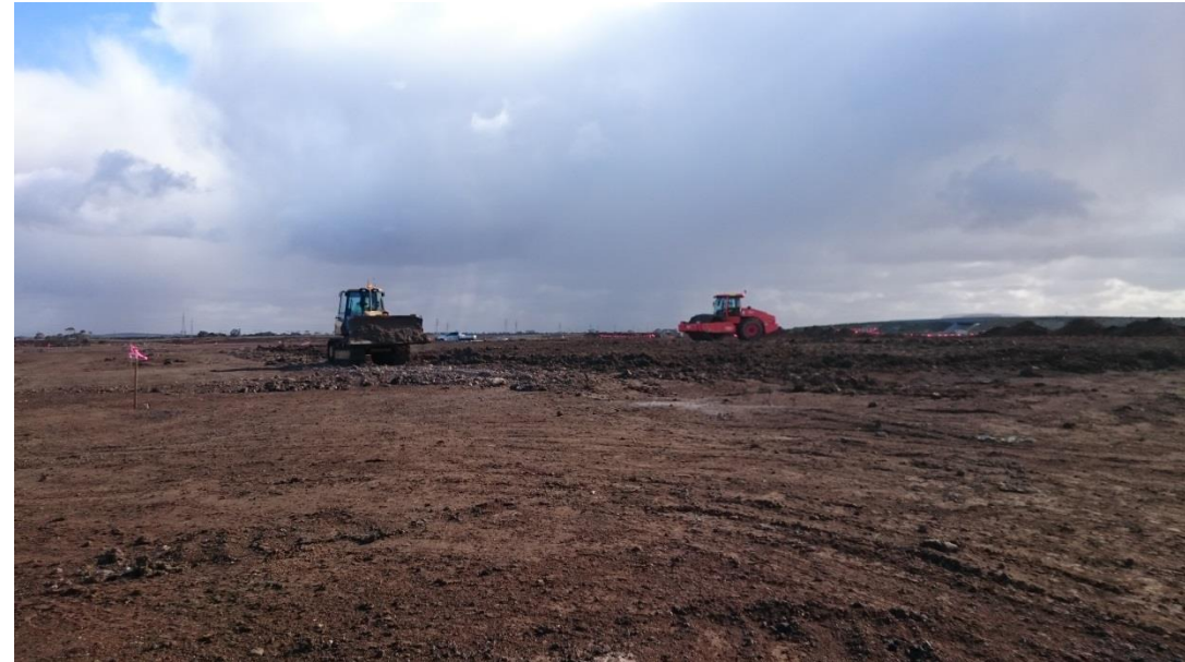
Stage 1: dozer placing more fill as part of layer 4 in grid I1 and I2
