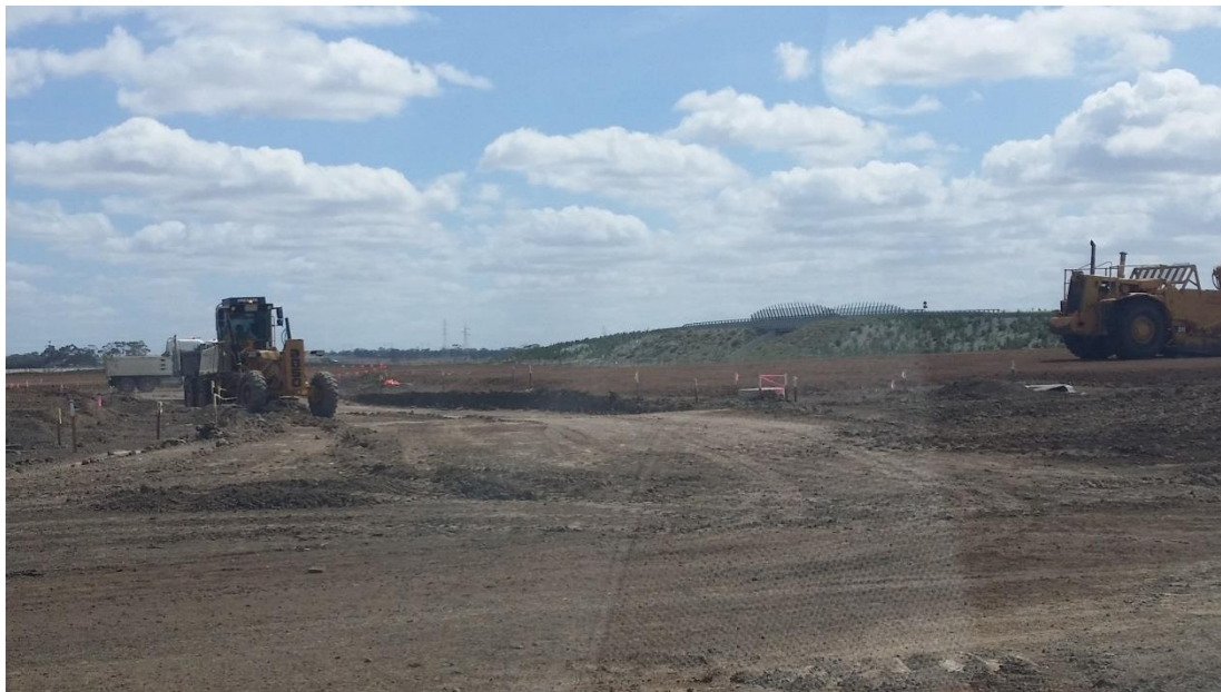
Stage 1: further grading of road E in grid M1 (E), M2 (E), N1 (W) and N2 (W)
