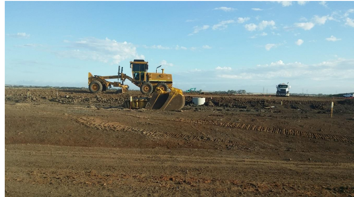
Stage 1: Grading of topsoil in grid L1 (E), L2 (E), M1 and M2
