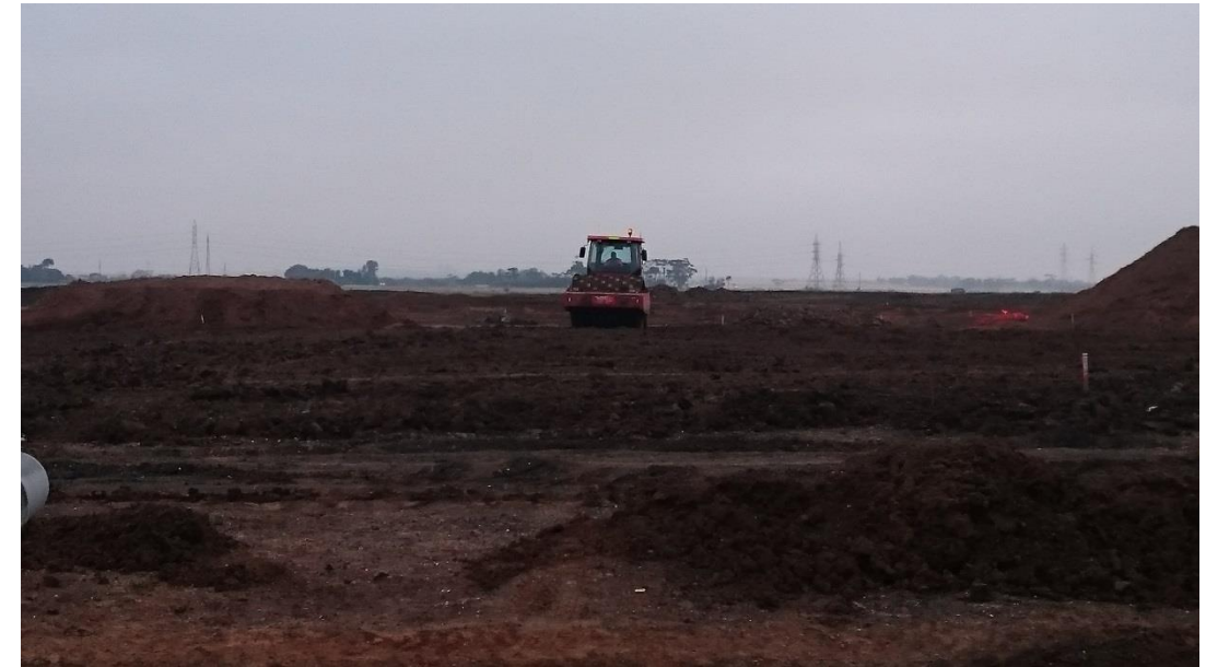
Stage 1: Pad foot roller being used to compact layer 6 in grid M2 prior to testing
