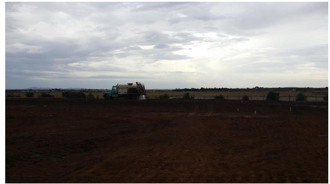
Stage 3: moisture conditioning of layer 2 material prior to placement of layer 3 in grid A5 (N) and A6 (S)
