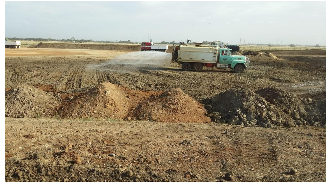
Stage 4: moisture conditioning of layer 1 material in grid L4, M4 and M5
