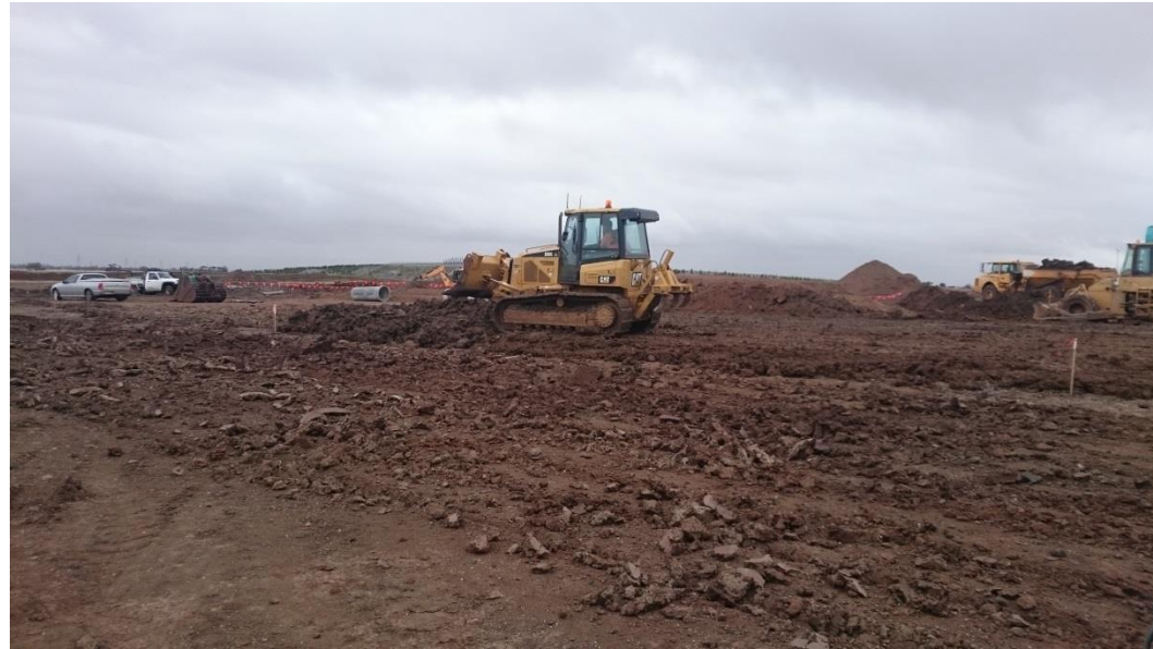
Stage 1: newly ripped section prior to placement of fill in grid K1 and K2 as part of layer 6
