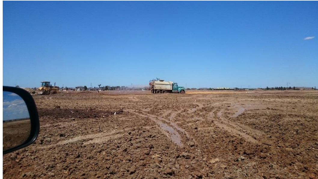
Compactor and Water cart moisture conditioning layer 2 in grid C5, C6, D5, D6
