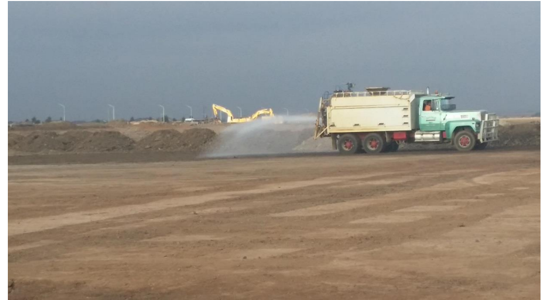
Stage 4: Moisture conditioning of subgrade and stockpiled material in grid N4 and N5
