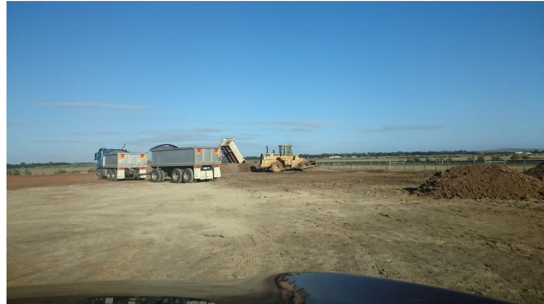
Stage 3: placing more fill as part of roadway in grid A6, B6 and C6
