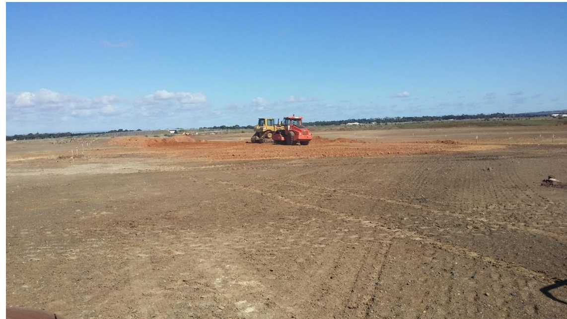
Stage 3: placement and rolling of fill material in grid H4 (W), G4 and F4
