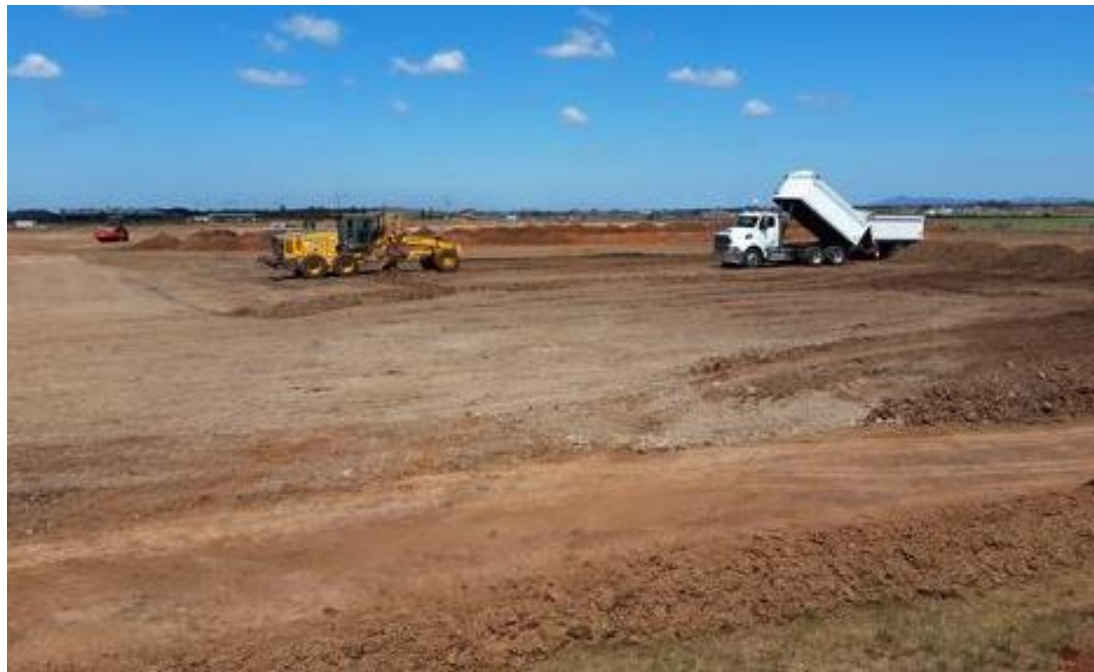
Grader placing layer 2 - C5 (north), C6 (south-west), B6 (south-east), and B5 (north-east).
