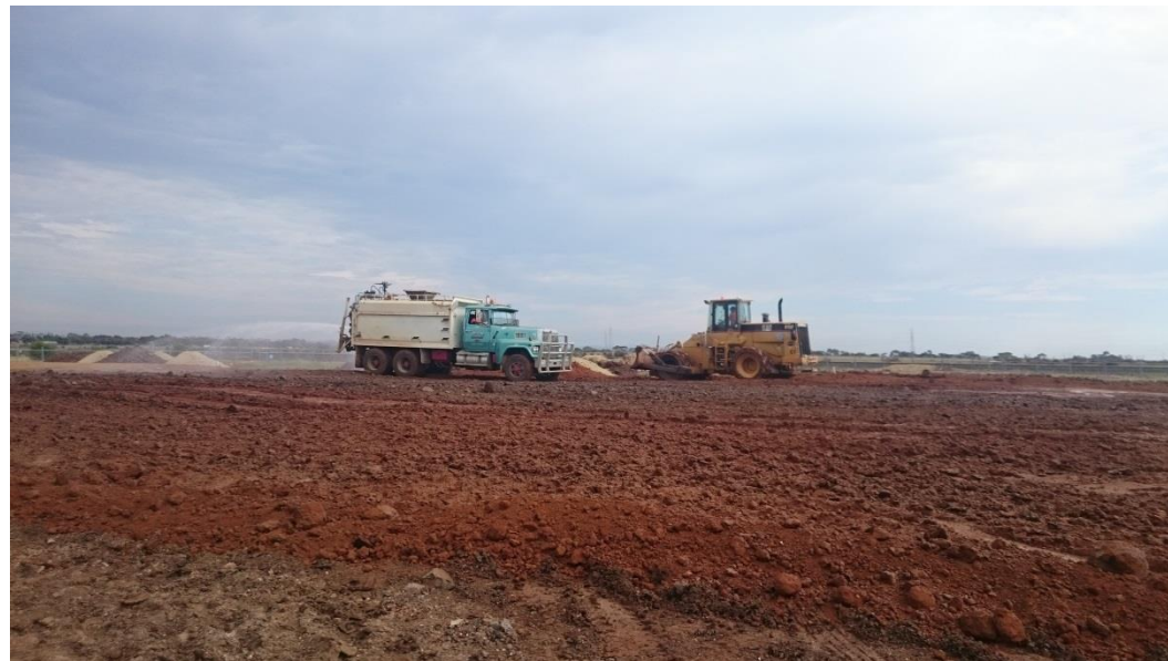
Stage 3: compactor placing layer 3 whilst being moisture conditioned in grid B5, B6, C5 and C6
