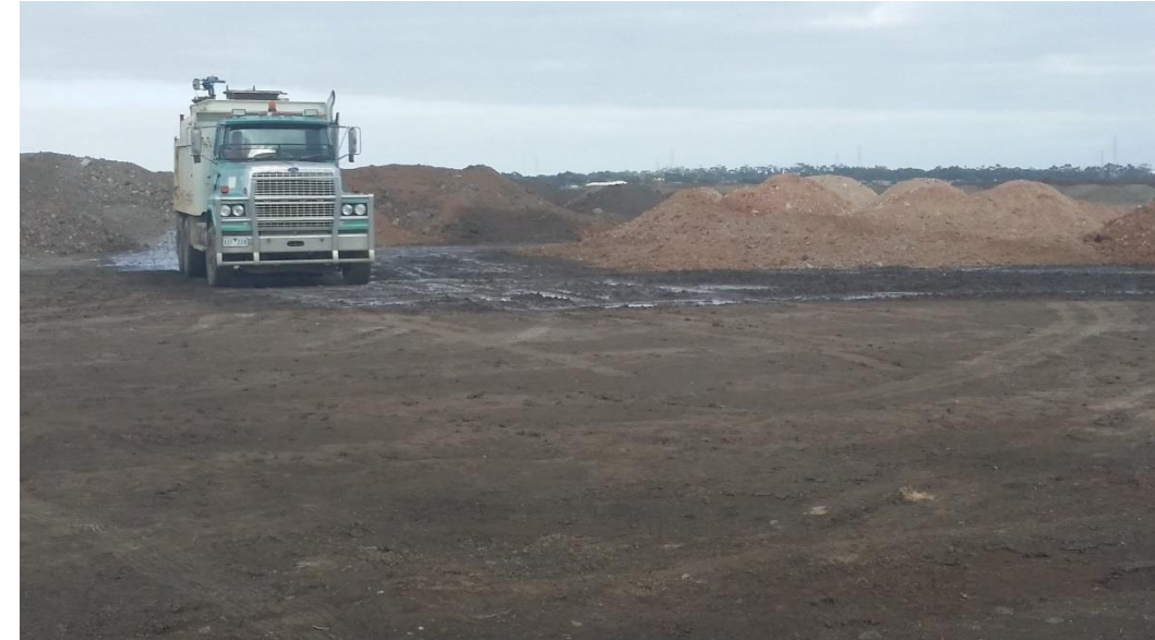
Stage 4: Moisture conditioning of subgrade prior to layer 1 placement in grid N3 (E), O3, O4 (E), and O5 (E)
