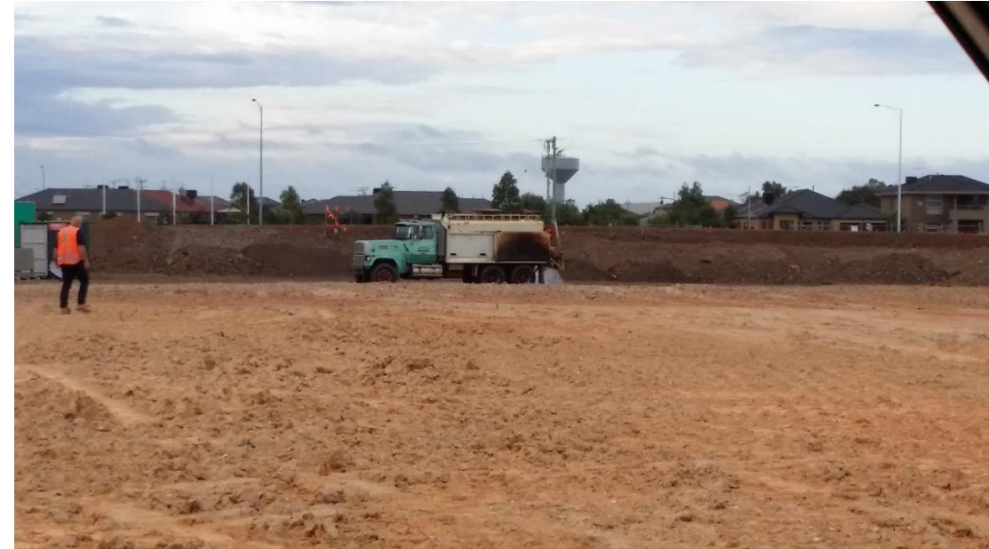
Stage 4: Moisture conditioning of subgrade prior to layer 1 placement in grid N2 (E) and O2
