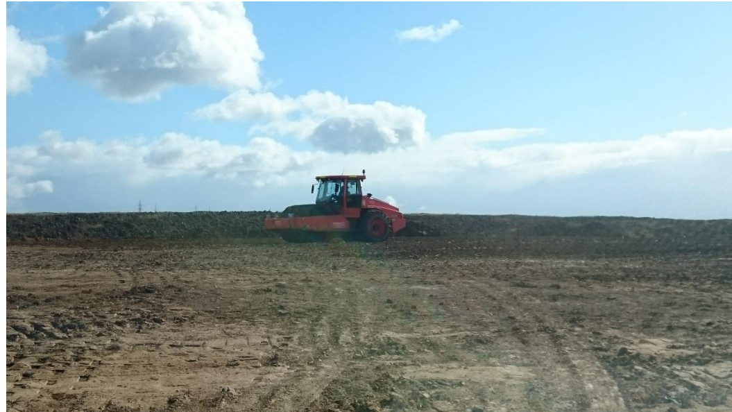
Stage 3: pad foot roller on layer 3 in grid G5 (W) and G6 (W)
