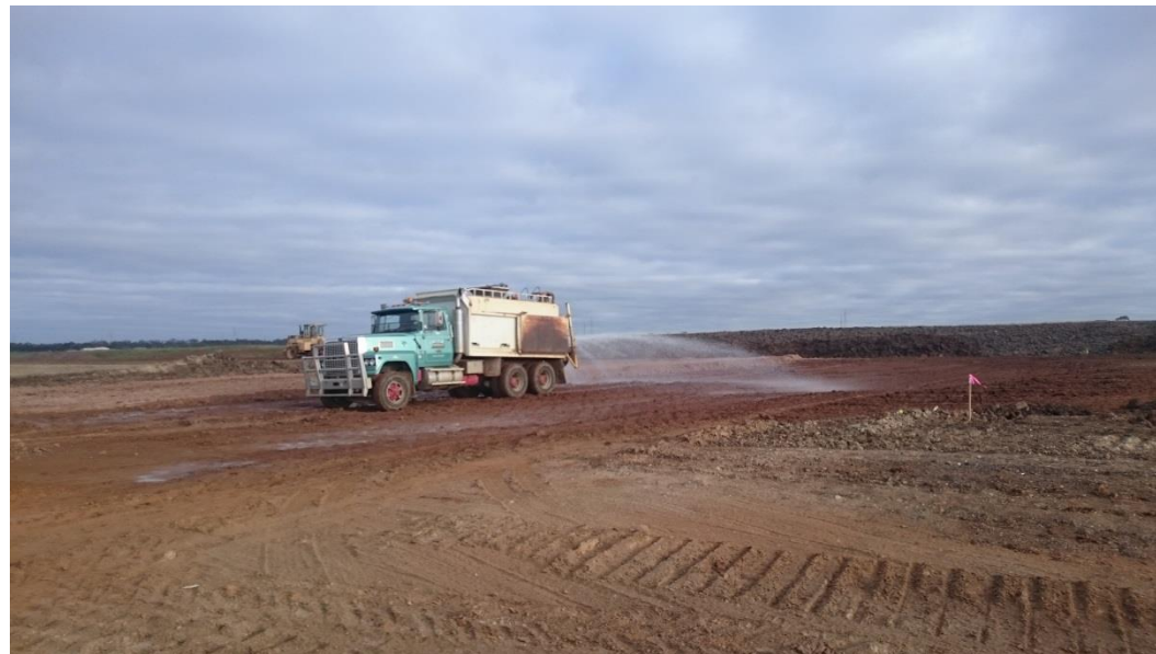
Stage 3: layer 3 being moisture conditioned in grid G5, G6, H5 and H6
