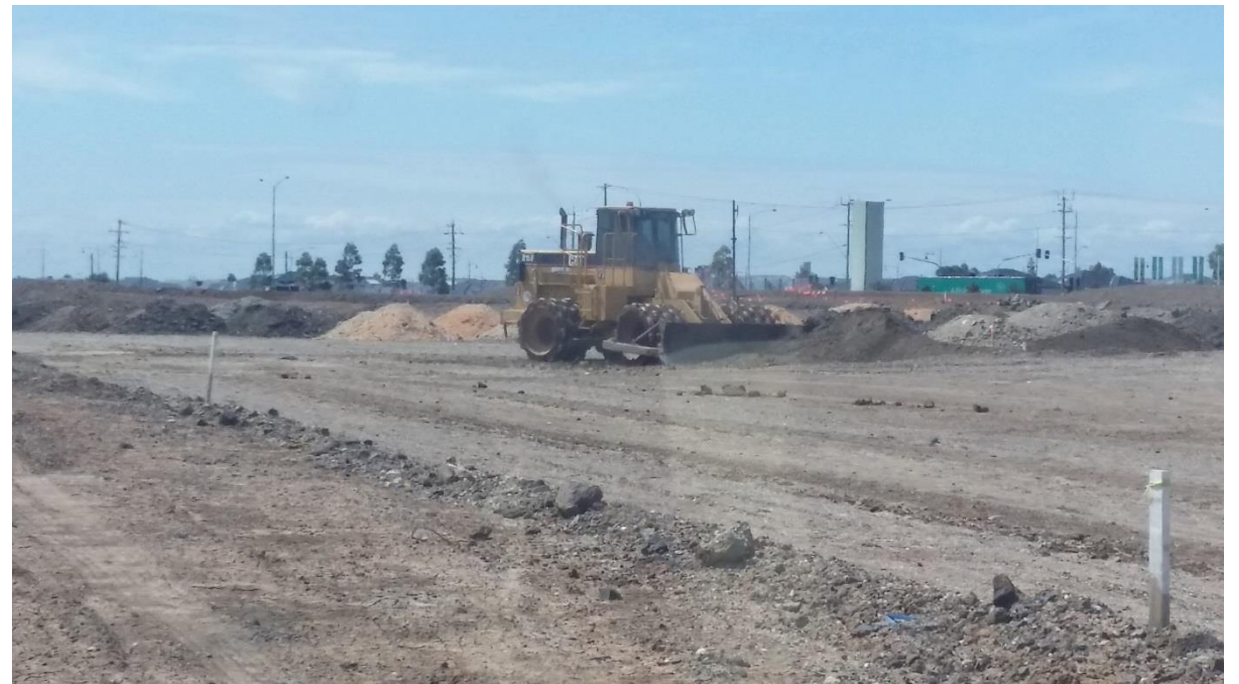
Stage 4: Displacement of stockpiles in order to assist with future layer placement.
