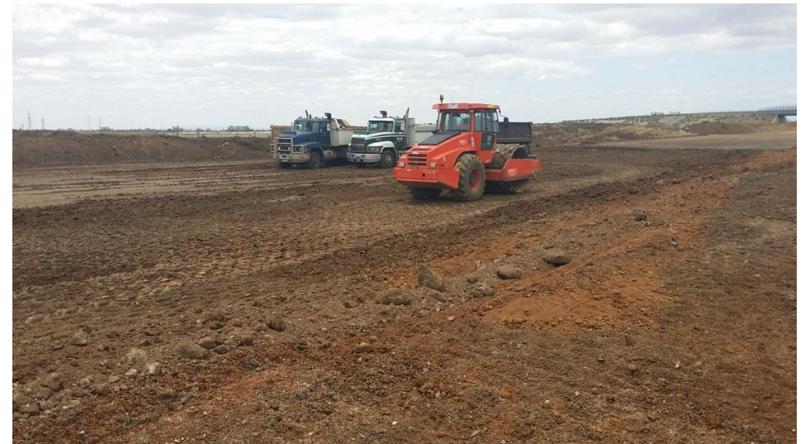
Stage 4: Layer 1 in grid H5 (NE), H6 (SE), I5 (N), I6 (S), J5 and J6 (S). Being rolled by padfoot roller.
