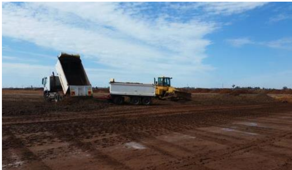
Dump Truck with trailer dumping imported fill ready for placement - grid column B
