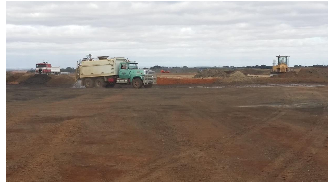
Stage 4: moisture conditioning of subgrade surface prior to layer 1 placement in grid L4 (N), L5, M4 (NW) and M5
