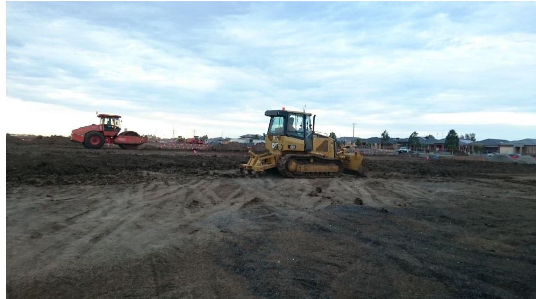
Stage 1: dozer placing more fill as part of layer 6 in grid I1, I2, J1 and J2
