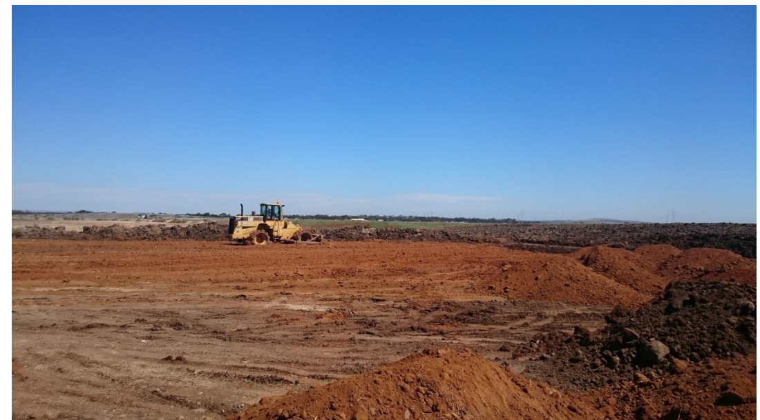
Stage 3: compactor being used on layer 1 in grid G5, G6, H5 and H6
