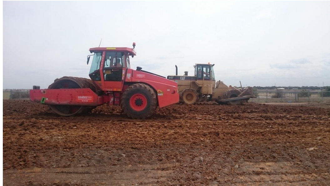
Pad foot roller and compactor on layer 3 in grid A5 and A6
