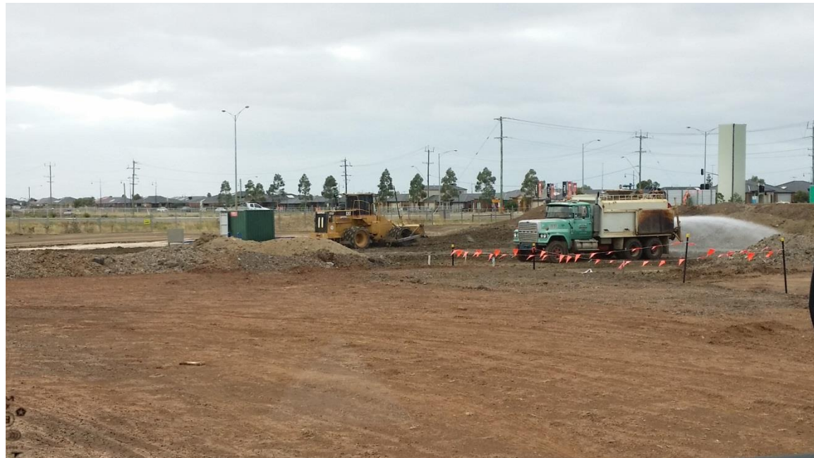
Stage 4: Moisture conditioning of placed layer 1 material in grid N2 (E) and O2.
