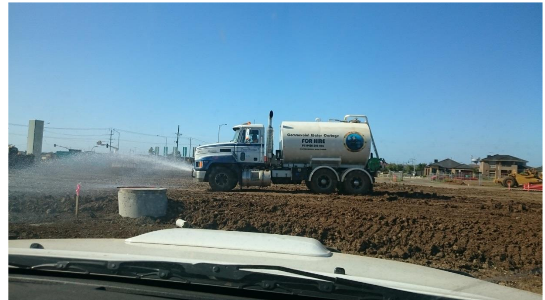
Stage 1: water cart moisture conditioning layer 7 in grid O1 (North) and O2 (South)
