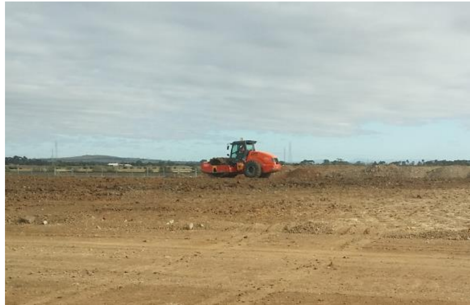
Stage 3: Rolling of layer 3 material in grid B5 (NE), B6 (SE), C5 (N), C6 (S), D5 and D6 (S)
