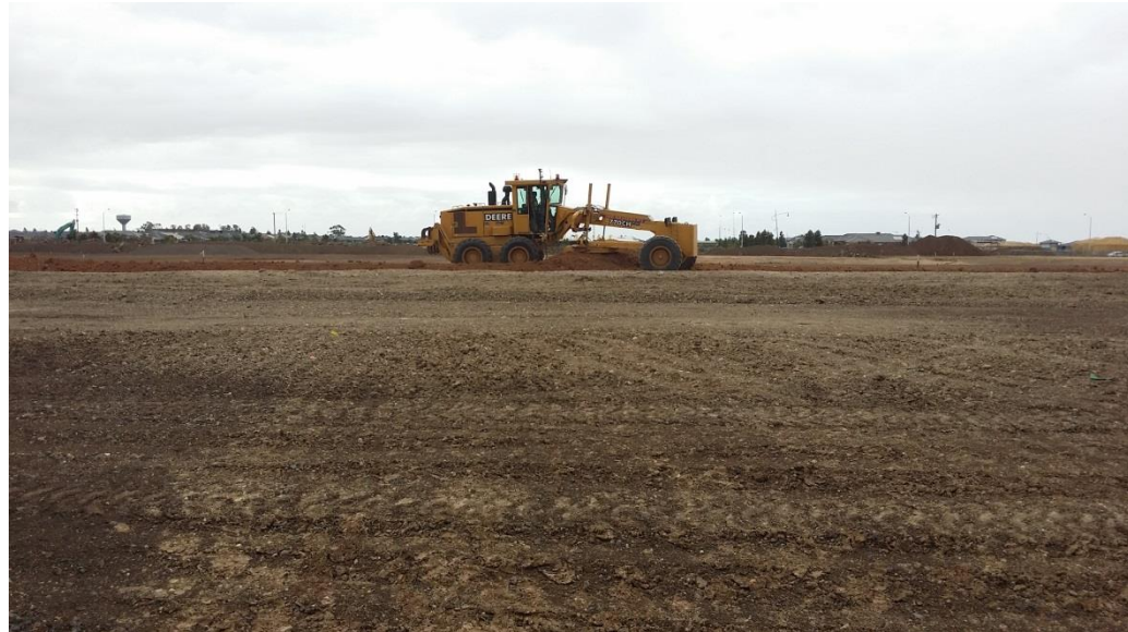
Stage 3: Spreading and grading to RL's in grid A4 (N), B4 (N) and C4 (N).
