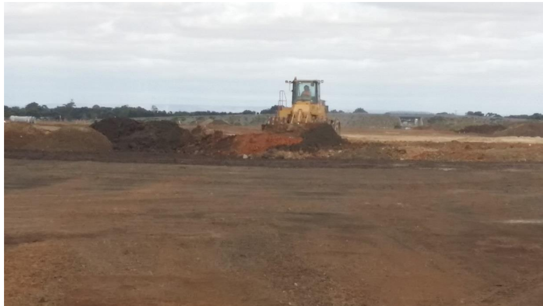
Stage 4: Placement and compaction of layer 1 material in grid L4 (N), L5, M4 (NW) and M5
