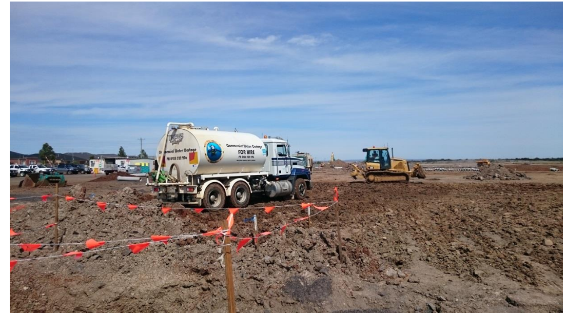
Stage 1: Water cart moisture conditioning ripped surface layer 6 in grid M1 and M2
