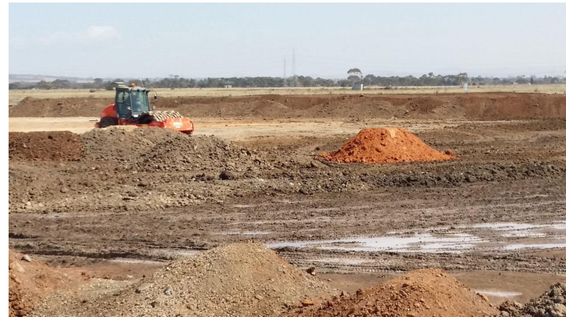
Stage 4: Rolling of layer 1 material in grid L4, L5, M4 and M5
