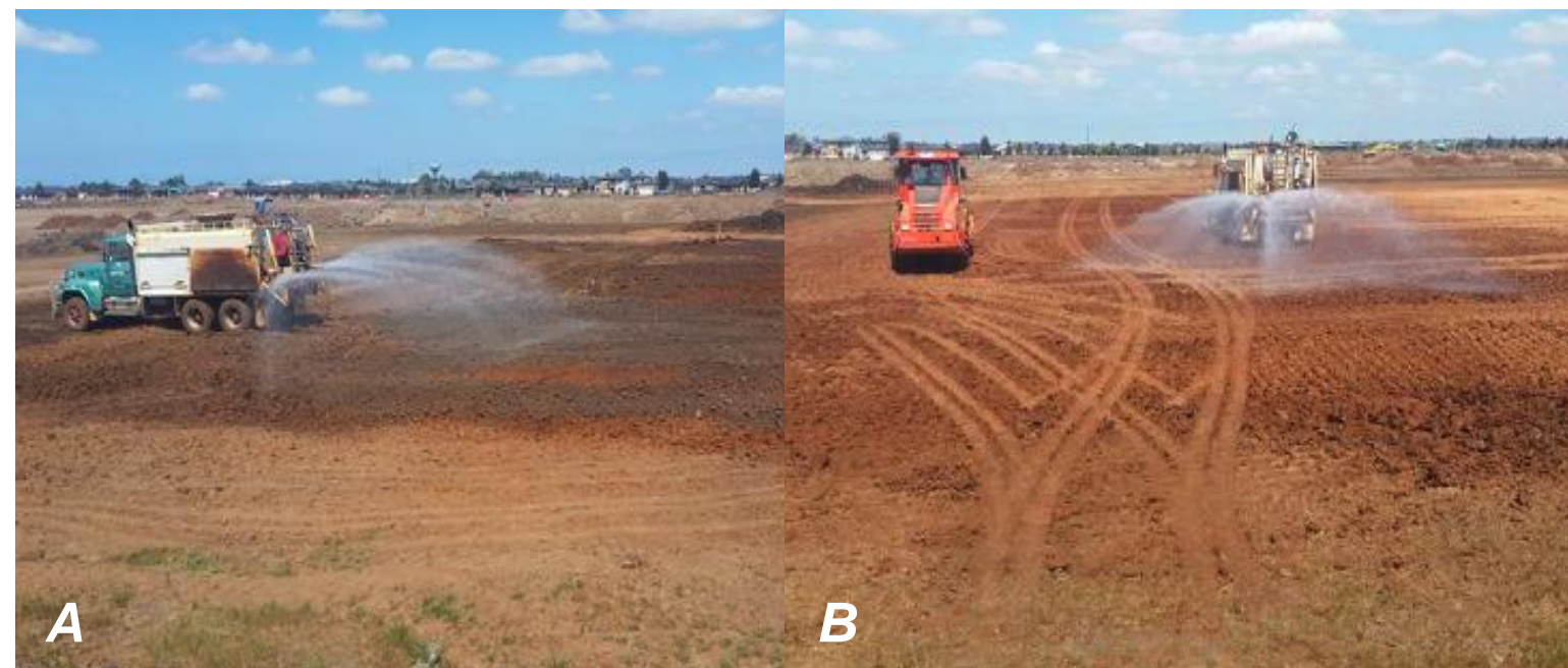
Water Cart moisture conditioning 100mm sublayer (A) - G6 (south-west), and layer 1 (B) F5 (north-east).
