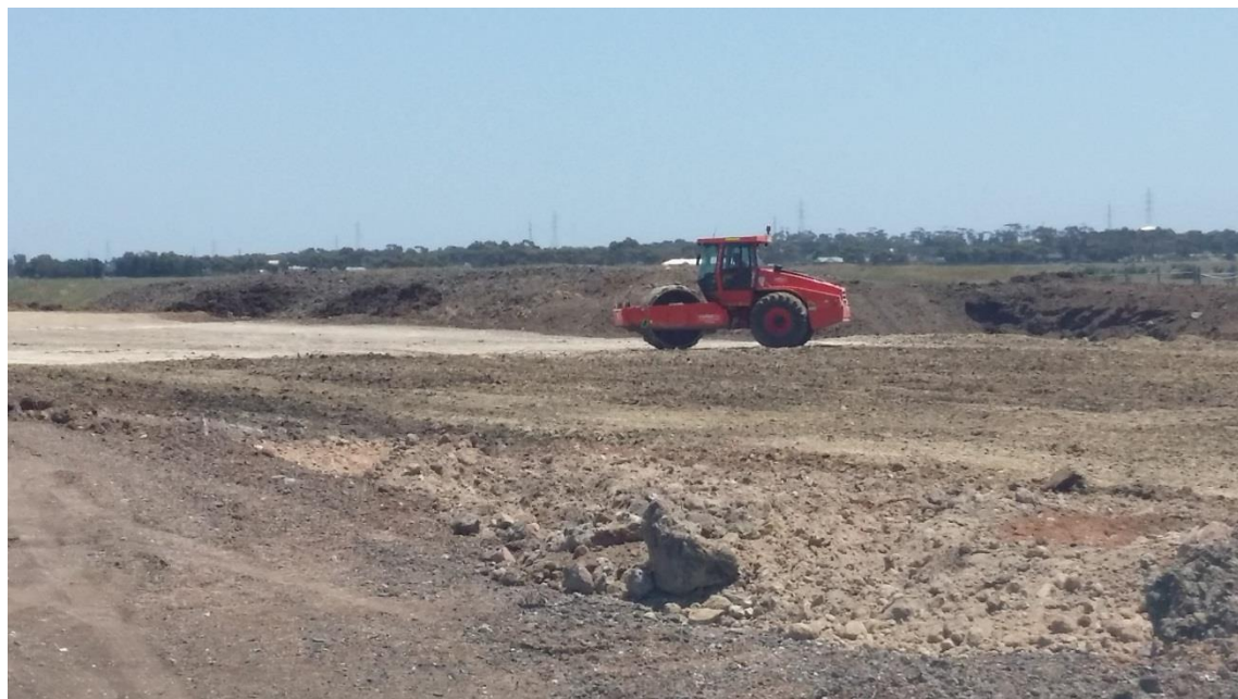
Stage 4: Rolling of layer 1 material by padfoot roller in grid J5 and J6 (S)
