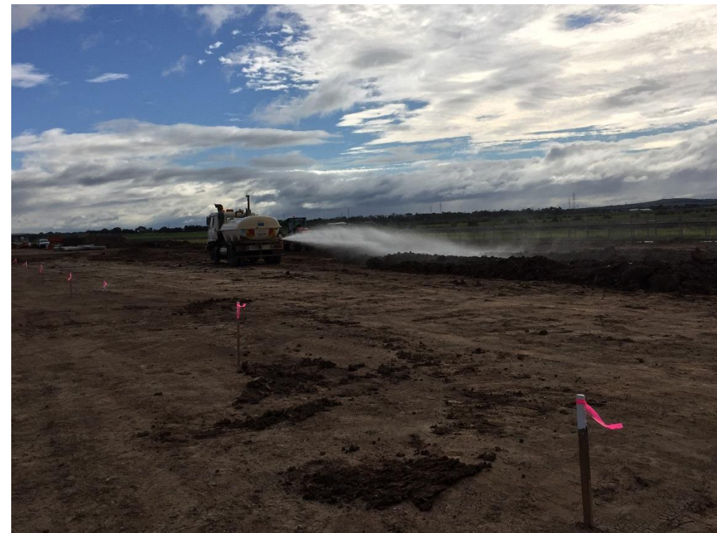
Stage 3: Water cart constantly maintaining moisture condition of fill stockpile during fill placement
