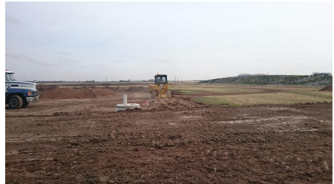
Stage 1: dozer ripping layer 6 prior to placing layer 7 in grid O2 (East) and water cart used for moisture conditioning
