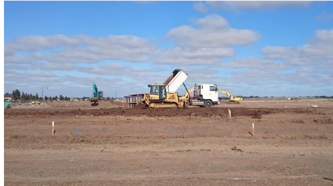
Stage 1: dozer placing more fill as part of layer 6 in grid I1, I2, J1 and J2
