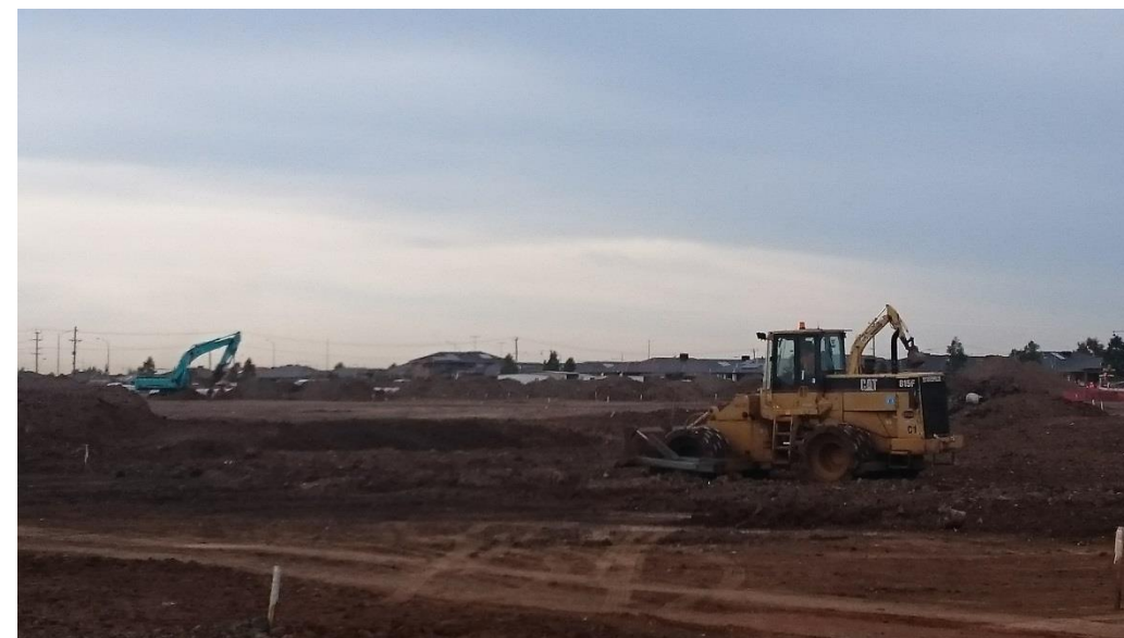
Compactor levelling fill from stockpile in layer 1 in grid G4 (Centre to East) and H4 (West, North-West and South-West)
