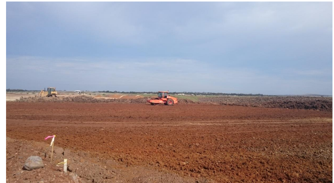
Stage 3: pad foot roller being used on layer 1 in grid G5 and G6 prior to testing
