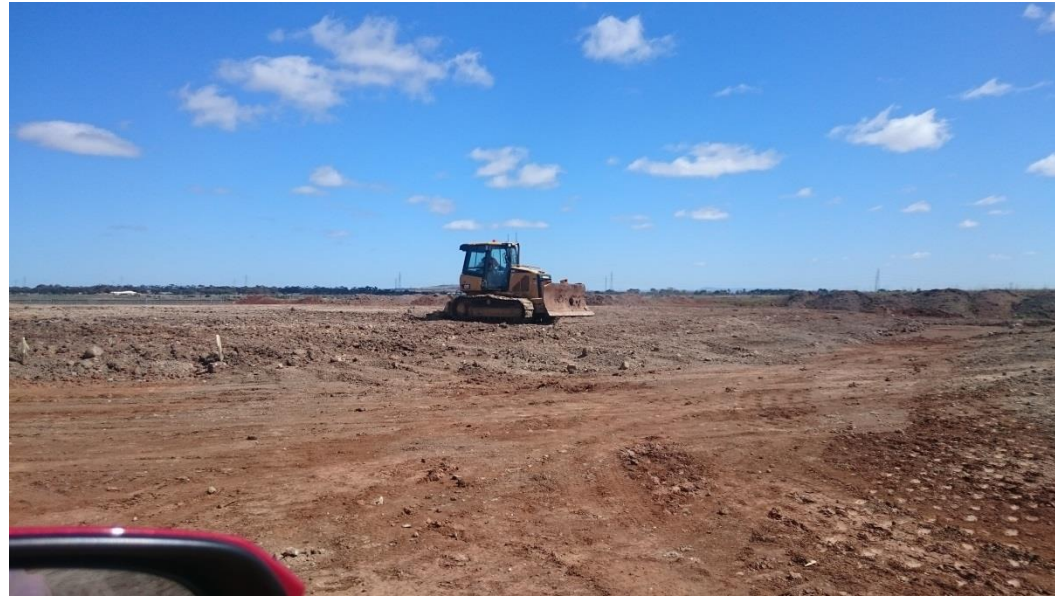
Stage 3: dozer ripping layer 3 in grid D5, D6, E5 (W) and E6 (W) to add moisture to layer
