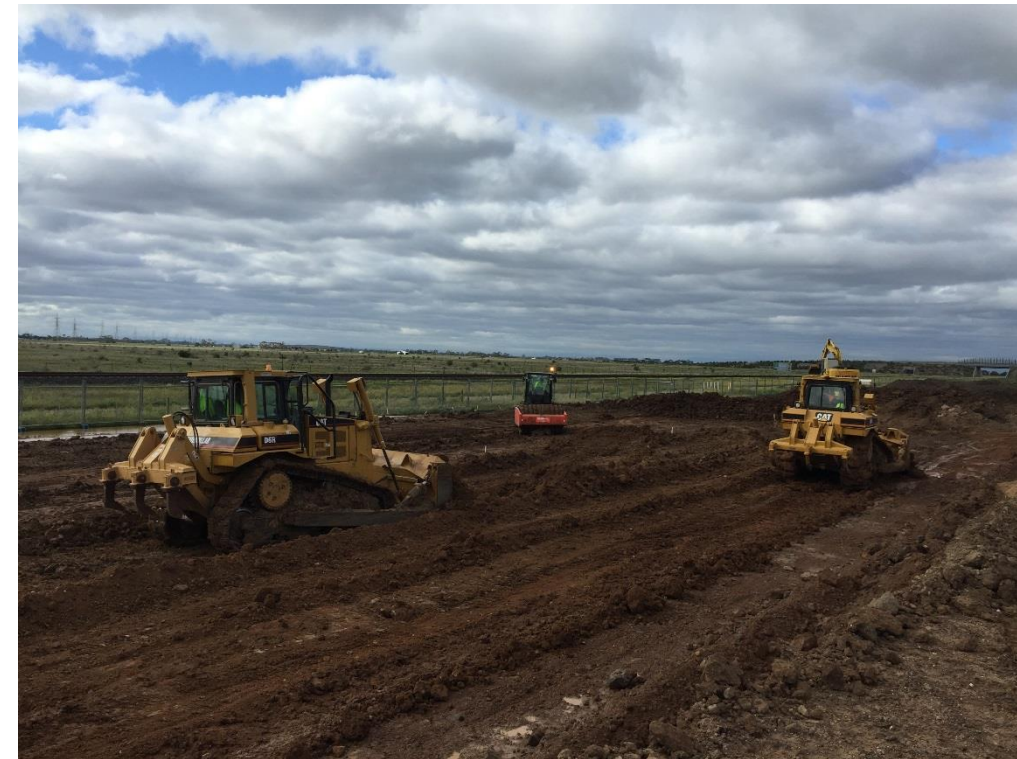
Stage 3: Dozers cutting two steps to key in the new engineered fill platform
