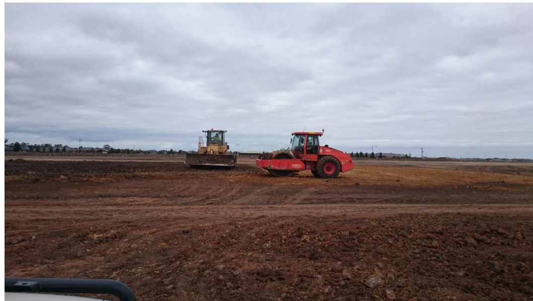
Compactor and pad foot roller on Layer 2 in D4, E4, F4 and G4
