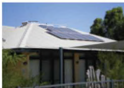
Solar PV system generating power from the sun (Source: Sustainable Mandurah Home)
