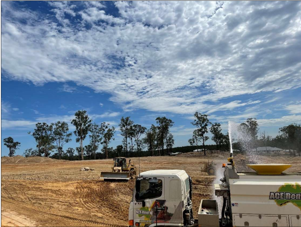
Figure 7 – Water cart working with compactor to condition and compact fill material. (Taken 7.12.2020)
