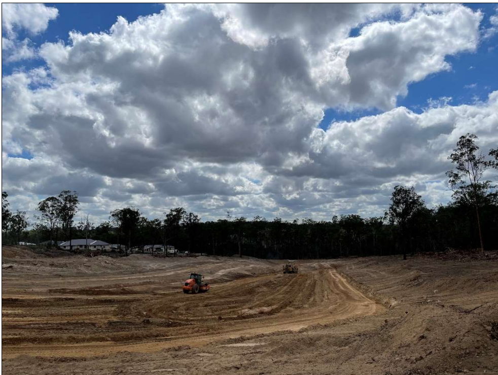
Figure 2 – Pad foot rollers working compaction on lower southern end of site. (Taken 27.11.2020)
