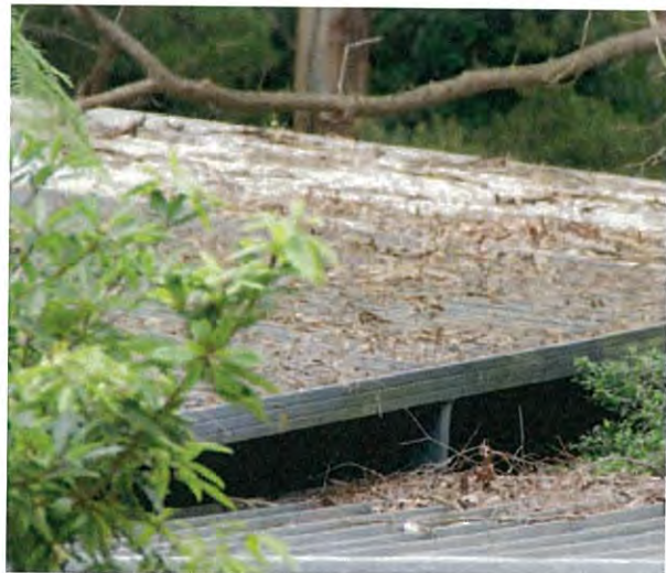
Vegetation located too close to a house poses a threat during bushfire.
